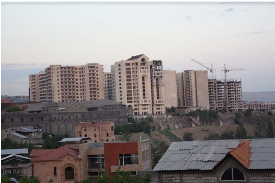
Construction of high-rise residential buildings in the site of former Yerevan fortress. Photo taken in August 2014 by the author.
