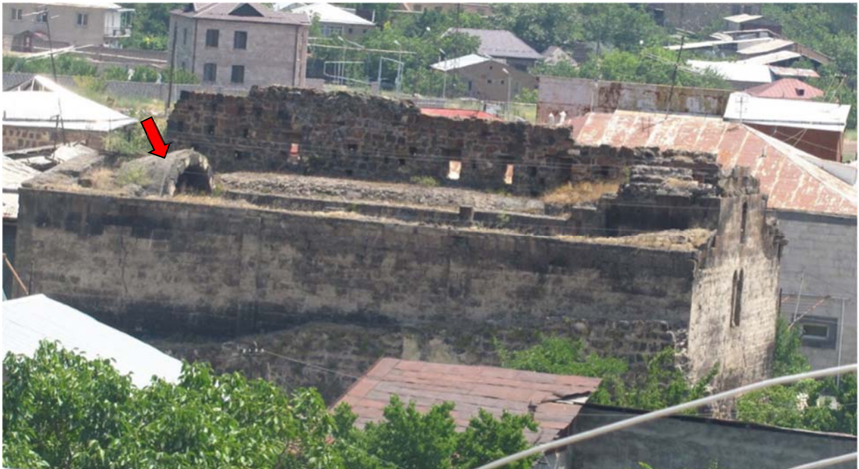
Tsiranavor Church. The reconstructed apse is covered by a steel reinforced concrete diaphragm during the 1963 restoration project.
