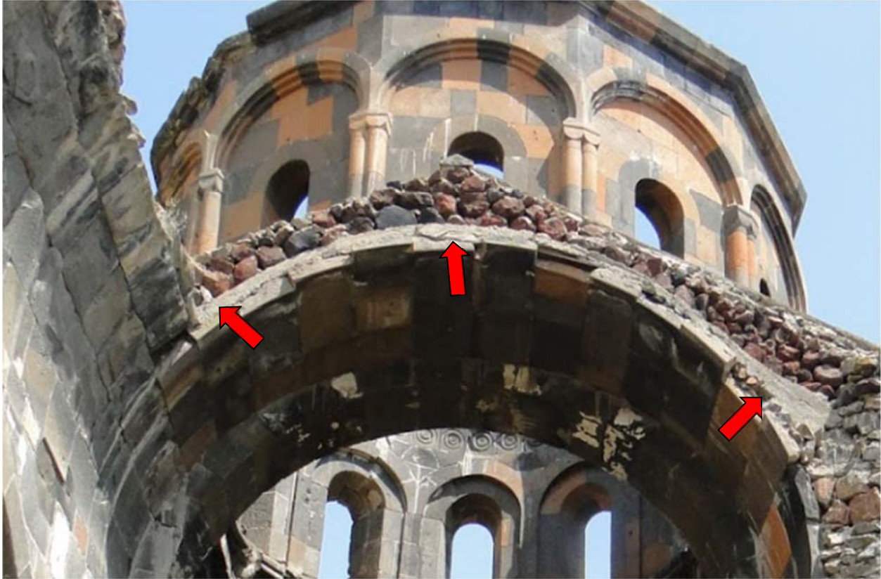
Talin Cathedral. Abundant use of concrete in consolidating the main arch supporting the dome is visible. Photo by Narek Sargsyan, August 2011.
