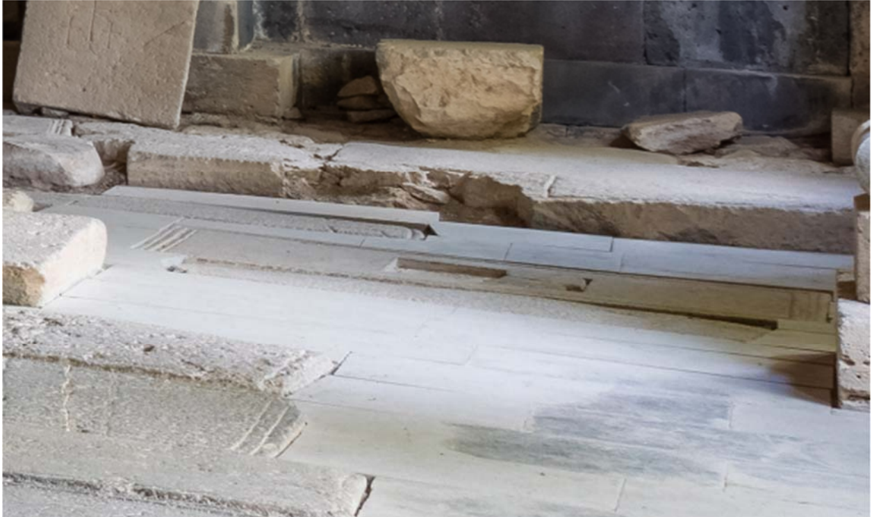
Despite its visual affect, the addition of the new pavement, so tightly next to the medieval tombstones will cause further damage. Photo taken on 30 September 2016 by Diego Delso.
