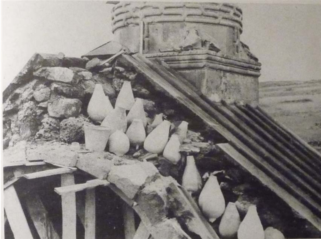
During the restoration activities of 1958, according to local traditional construction techniques, clay pots were used in decreasing the load of the masonry between the vault and the roof.
