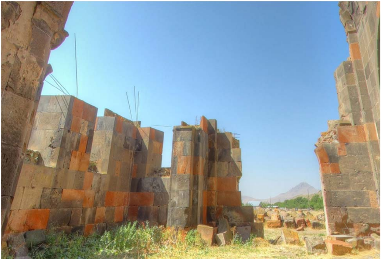
Talin Cathedral. Using steel reinforced concrete in restoring destroyed walls are visible. Photo by Seda Khachatryan, November 2015.
