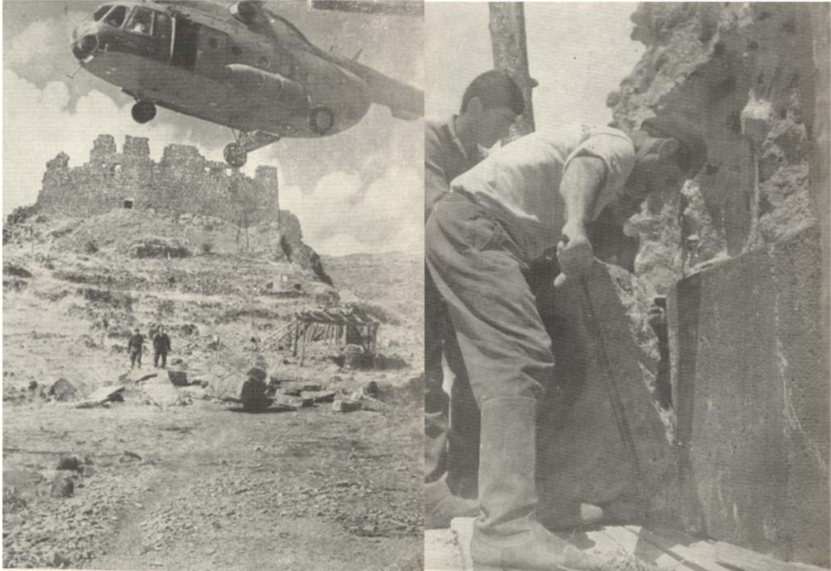
Left: Using Helicopter to bring the masonry to the site. Right: Stonemasons installing a stone block.
