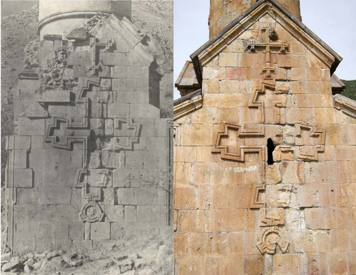
The eastern elevation of Surb Astvatsatsin Church in Spitakavor Monastery. Left: Before the restoration project of 1970-71. Right: Current situation of the eastern elevation. Photo by Vardan Mikayelyan taken in June 2017.
