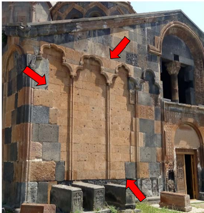
The new stones used in 1948 restoration project are easily recognizable. Photo by Hasmik Martirosyan, July 2017.
