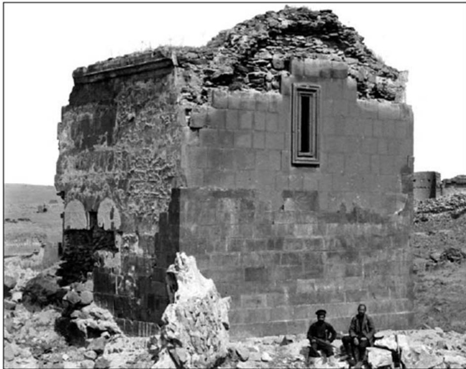
Figure 9: Top: The Armenian Chalcedonian church named “Georgian” from the north-east before its partial restoration implemented in 1904 (photo 1900-1904). Bottom: The same church after the partial preservation. Photo between 1904-1910. Photos from Karapetyan, Samvel. Ani-1050 , Yerevan: RAA, 2011, p. 211.
