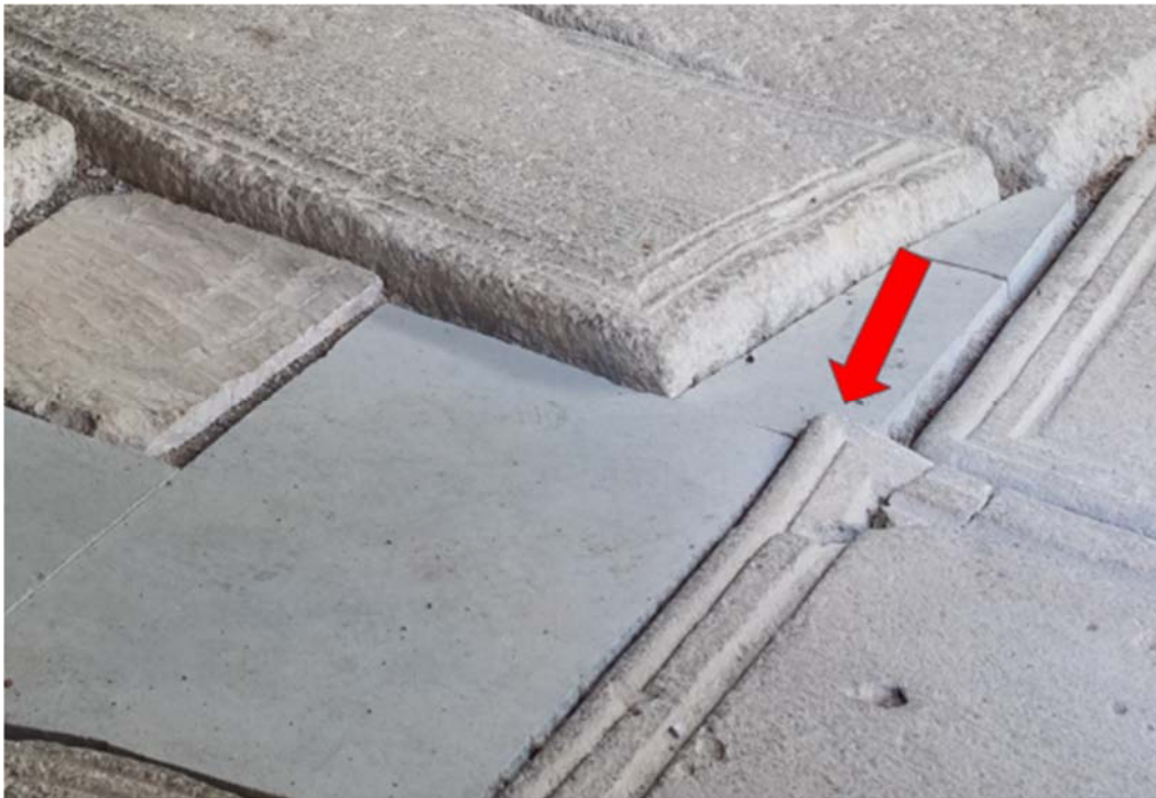
A close-up view of the new pavement, pointing out the damage caused to the medieval tombstones in Sanahin Monastery, one of the three World Heritage Sites of Armenia. Photo taken on 30 September 2016 by Diego Delso.
