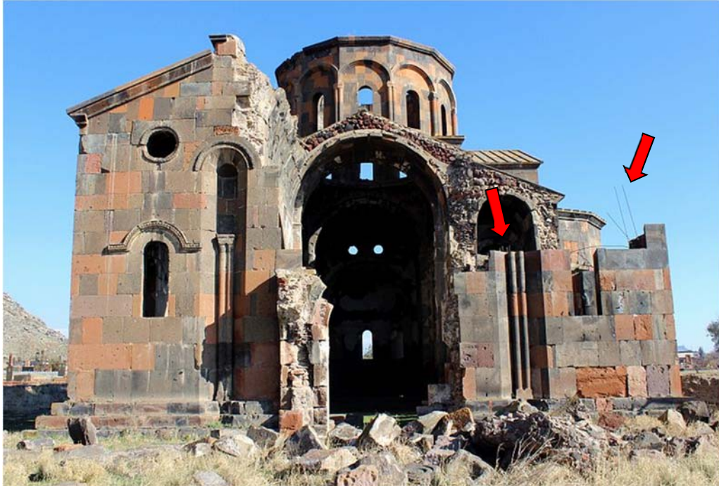
According to the policies of the time, large amount of steel reinforced concrete was used in consolidating the loose masonry. Concrete was used as a more high tech alternative for traditional lime mortar. The remainings of protruding steel rods are still visible in various parts of the monument. Photo taken by Travis K. Witt in November 2016.
