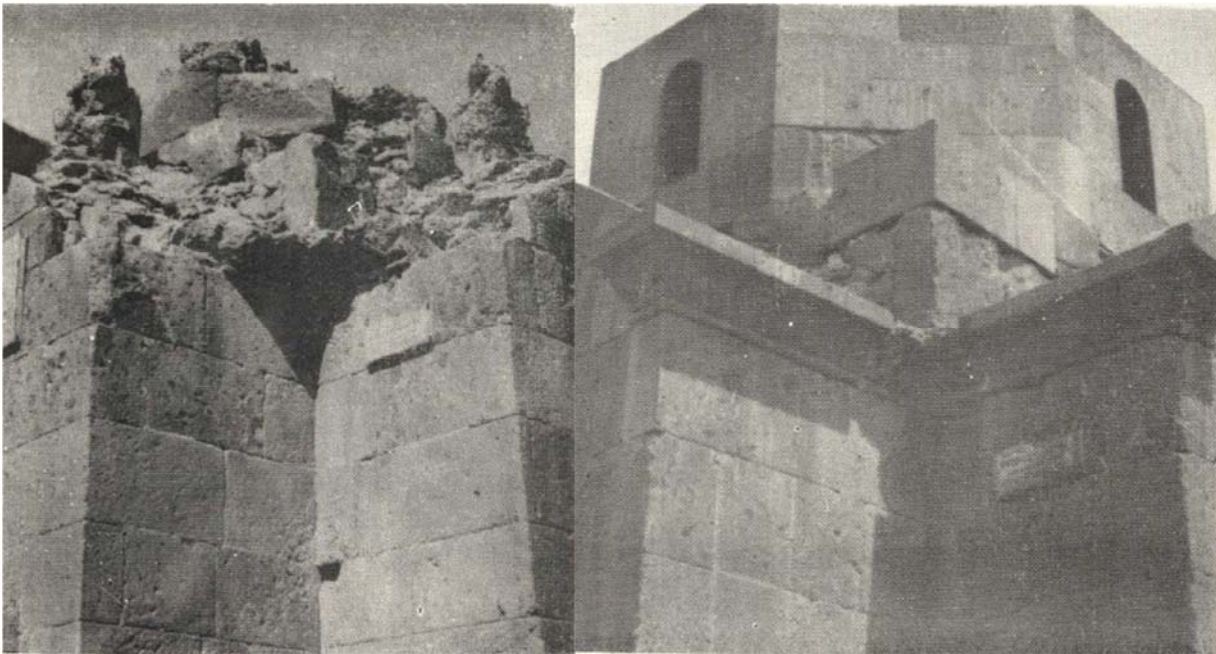
The cornices and drum of Surb Sion Church before and after the restoration project of 1950.
