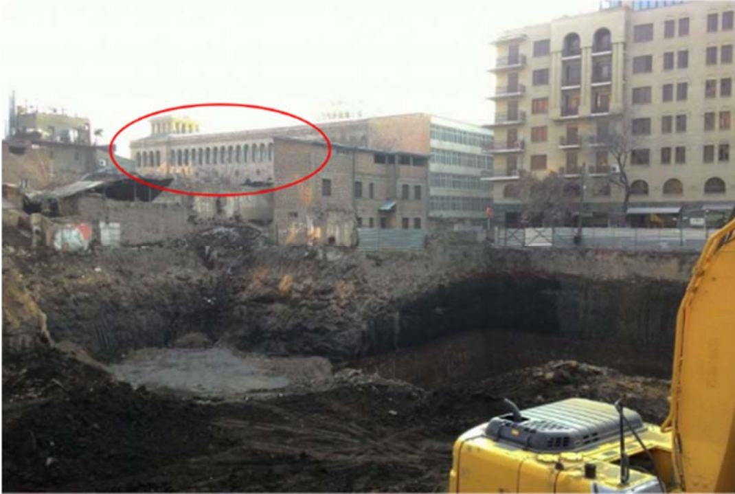
The area of Old Yerevan project. The building around the Republic Square is visited on upper left and the remaining old structures which are going to relate to the project are visible in the middle of the photo.
