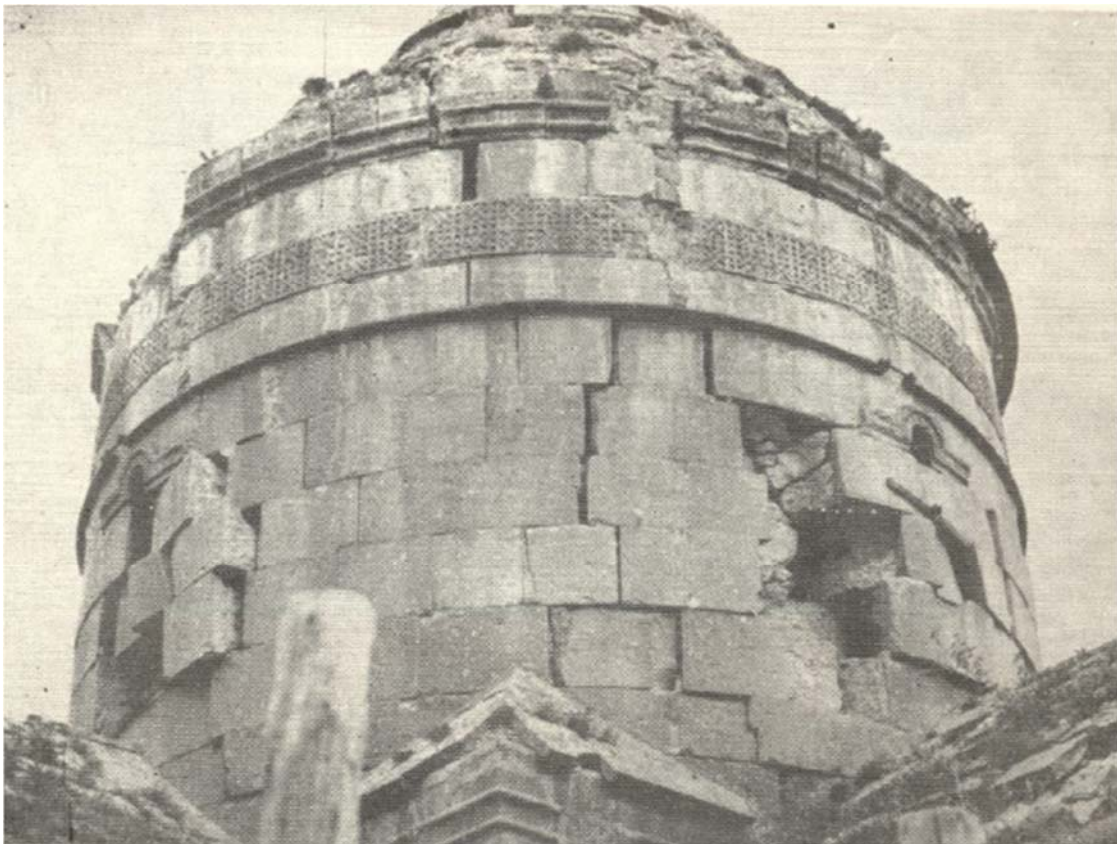
The drum of Surb Astvatsatsin Church in Goshavank before the restoration project of 1957-59. A large amount of the original basalt stones are standing but in verge of collapse.
