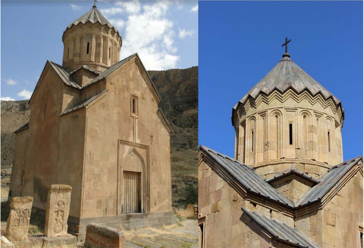
Current situation. A brand new stone dome, not recognizable from the original construction is added in 1998. Photo by Narek Sargsyan, October 2014.
