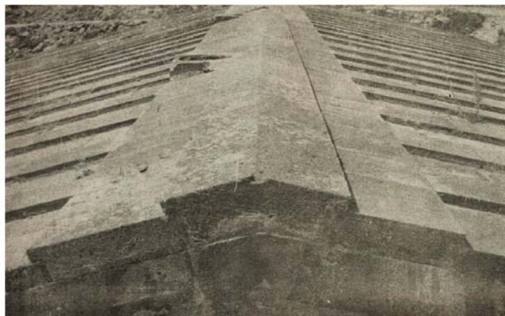
Detail of the restored roof of Selim Caravanserai after the restoration project of 1955-59.
