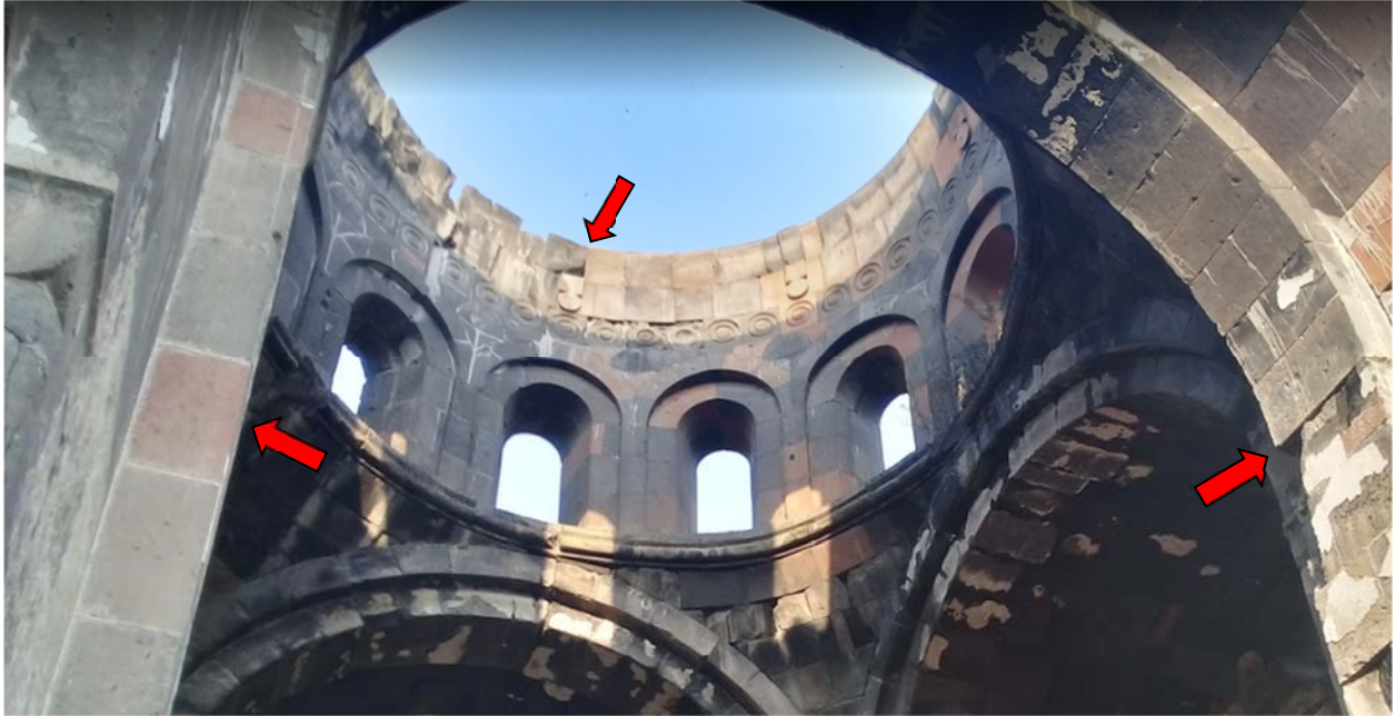
Talin Cathedral. The drum is completely reconstructed. The difference between the original and new masonry is highlighted. Photo by Arman Barseghyan in August 2017.
