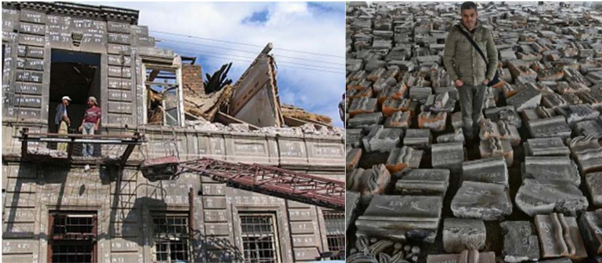
Left: Dismantling the facade of a nineteenth century stone building in hope of rebuilding it in a new location. Right: Hayk Bianjyan at the store of the dismantled building. Photo taken by Lena Nazaryan.
