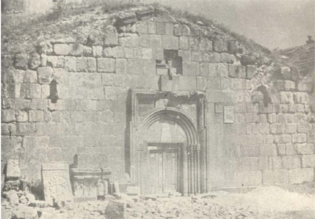
The western elevation of the narthex, Surb Astvatsatsin Church in Goshavank before the restoration project of 1957-59. The stone blocks on upper levels are heavily damaged, the roof needs to be repaired and some stones are missing.
