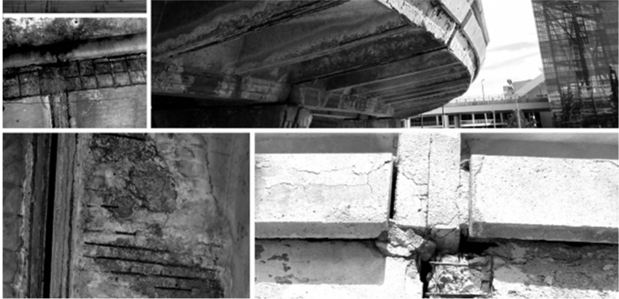
The decayed concrete structure of the old Zvartnots terminal.
