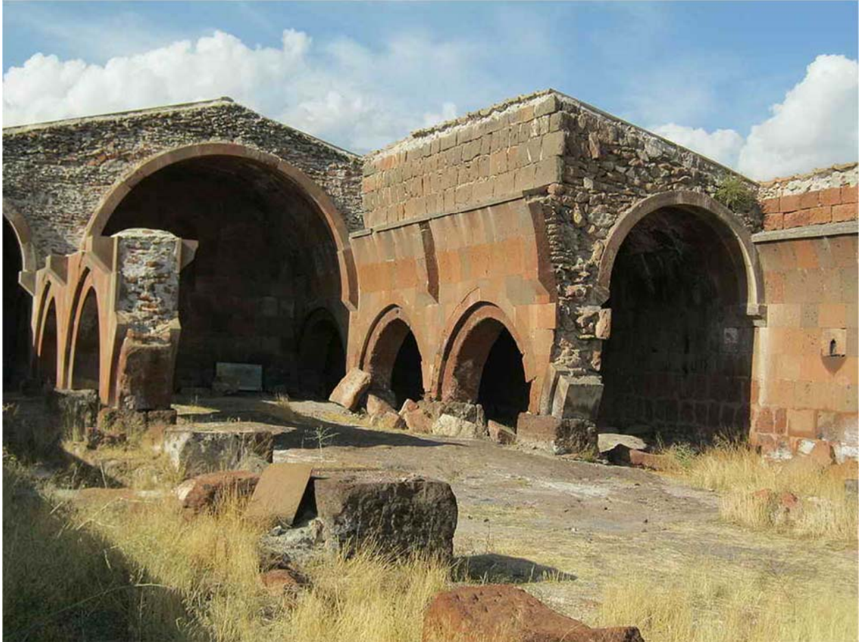
Talin Caravanserai with recently added segment of the main vault. This is an interesting example of preservation project which other than the grandeur of the building, clearly shows the construction techniques and materials. Photo by author, August 2014.
