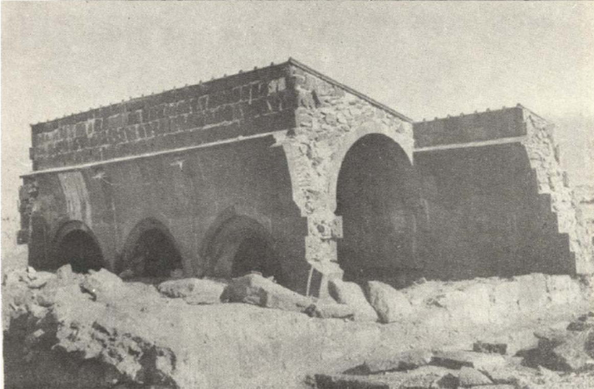
Talin caravanserai before and after the restoration project of 1956. The side vault is reconstructed and covered by a roof.
