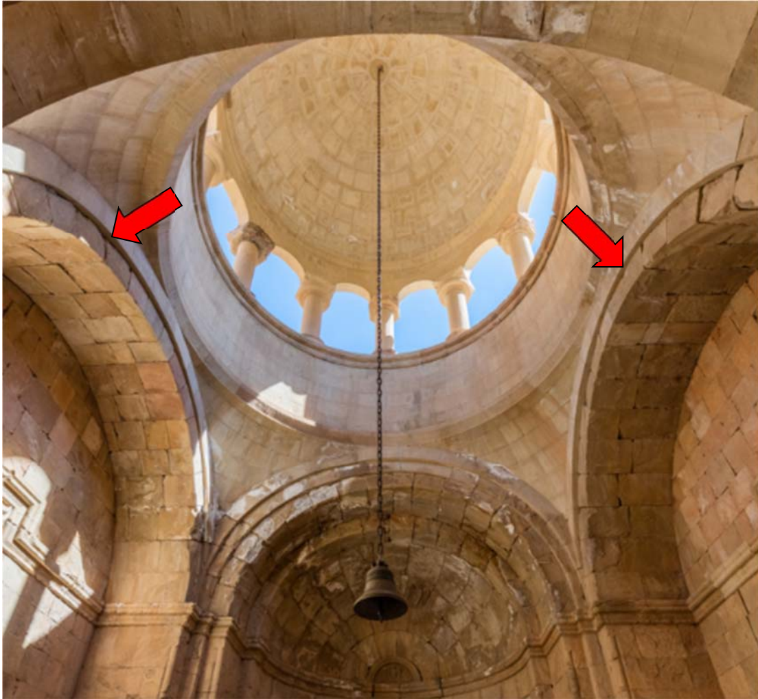
Interior view of the recently constructed rotunda in Surb Astvatsatsin of Noravank. The new arches are resting upon the old ones. Photo by Diego Delso.
