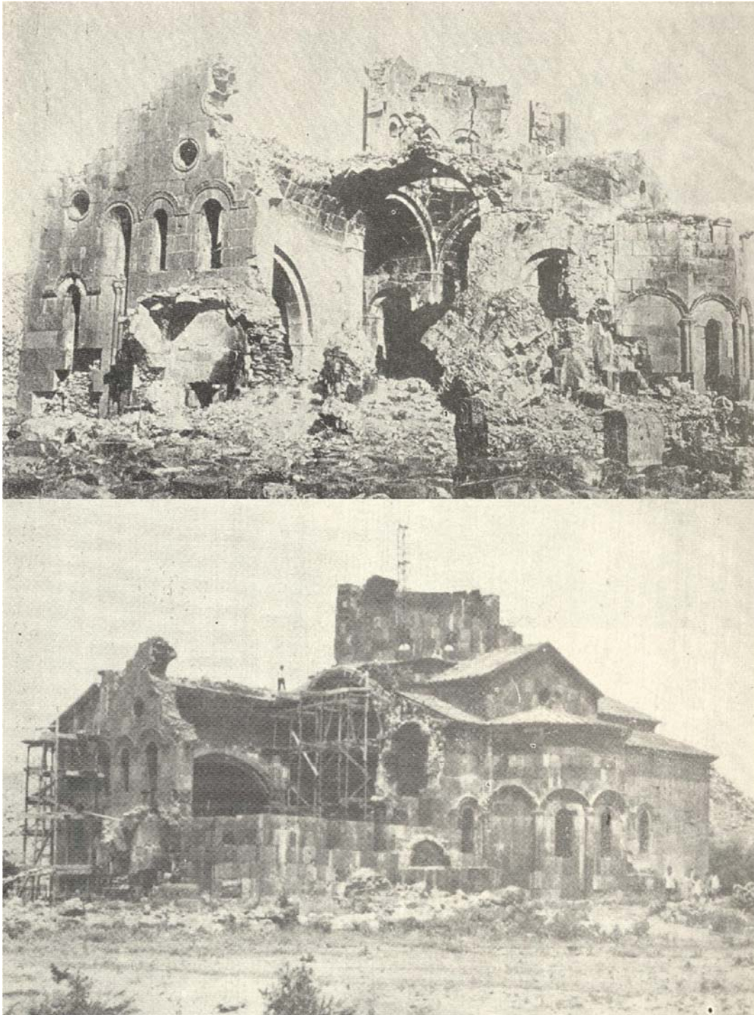
Talin Cathedral before and after the restoration project which took place in various phases between 1958 and 1980. The project mainly concentrated on consolidating the loose masonry, restoring the missing stones, pediments, and roofs. The monument was heavily damaged, therefore, they did not cover the nave neither construct the drum and dome.
