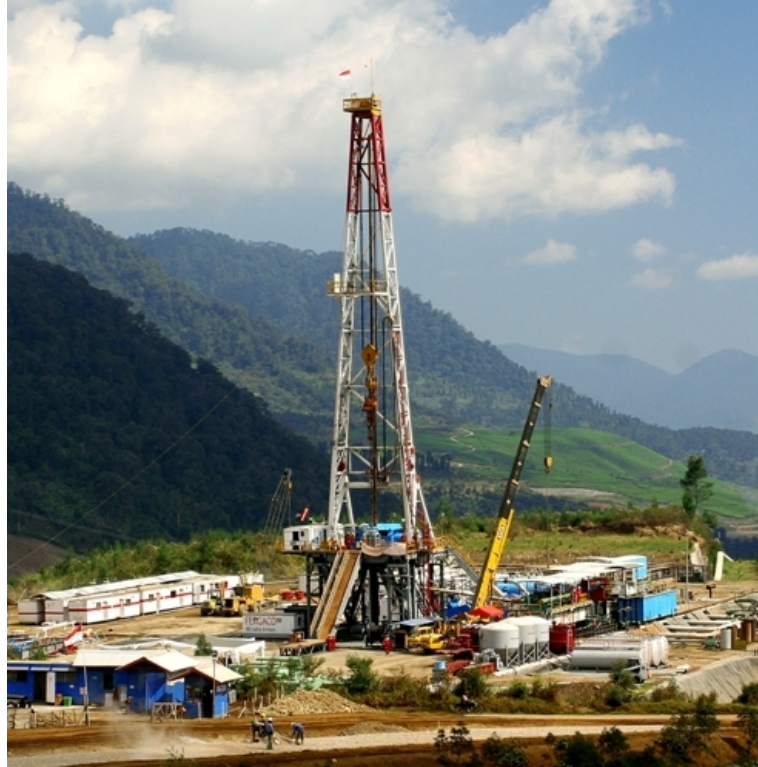
Figure 4.4: Onshore extracting well
