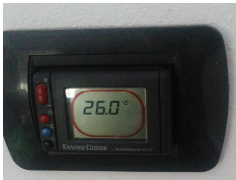
Figure 10 Room temperature (Higher Ambient)
