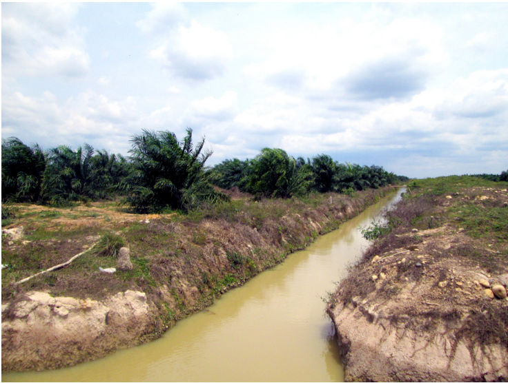
Water drainage system
