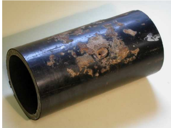
Fig 1.6 – Stray current corrosion on a coated carbon steel pipe
