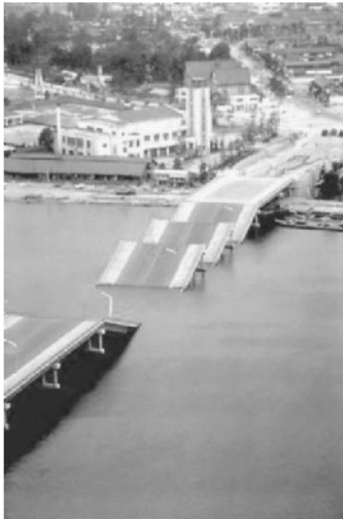
Figure 1-1 Collapse of the Showa Bridge during the Niigata earthquake on June 16, 1964. (Photograph from the Godden Collection, EERC, University of California, Berkeley.)
