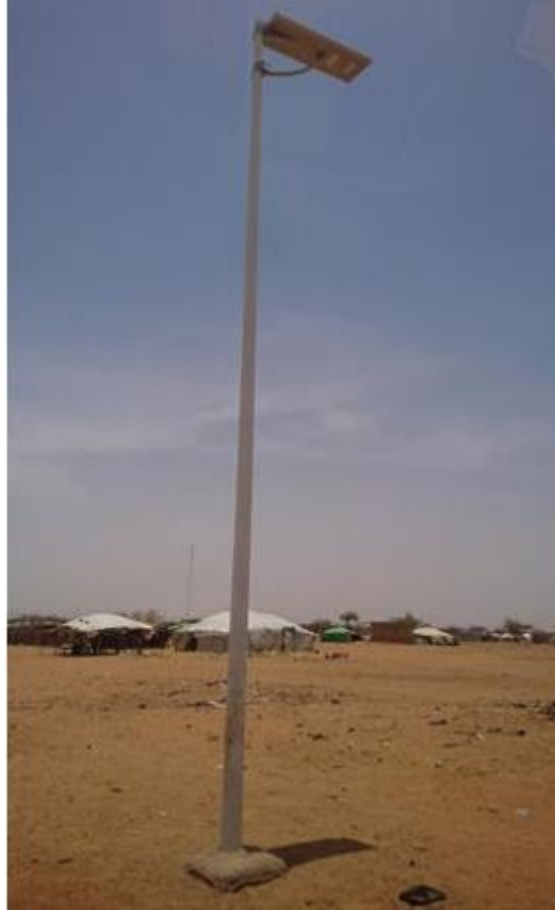
Figure 29 - Solar Street Lighting in Goudoubo Refugee Camp. Source: [30]
