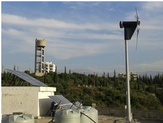
Figure 3.29 PV array and wind turbine on the rooftop. Credits: the Author.
