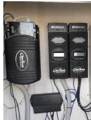
Figure 3.30 Inverter and MPPTs. Credits: the Author.
