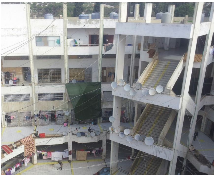
Figure 3.15 View of the inside structure of the building, giving evidence of the precarious conditions of the electric system. On the roof, the water tanks are visible. Credits: the Author.
