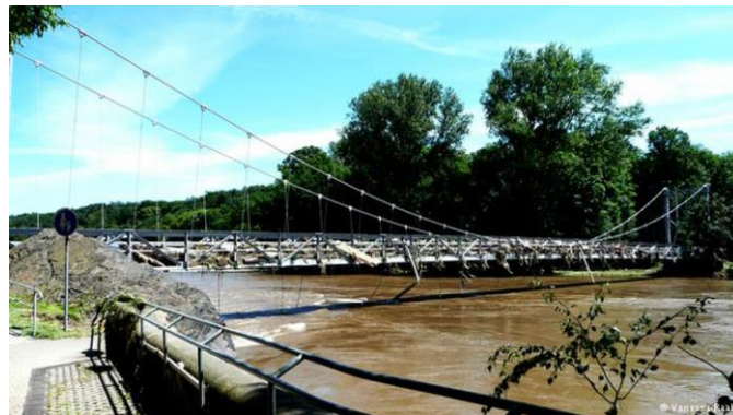
Figure 46 Suspension bridge covered in debris on June 6 th , 2013 (source: DW, 2013).
