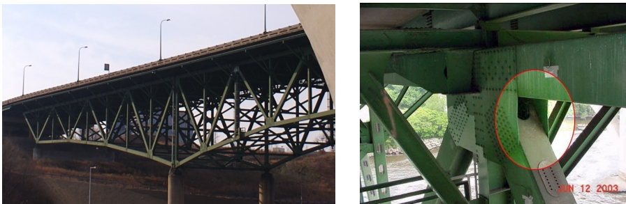
Figure 3.2: Mississippi River Bridge in Minneapolis and the gusset plate collapsed in 2007.
