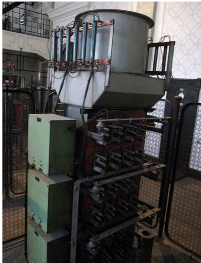
Figure C.20: Solid-state substation diode rectifier, commissioned in 1960s, now dismissed (Novate Milanese, Italy. Source: delta-november.it).
