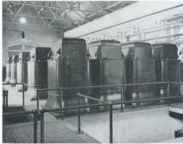
AIR-BLAST TRANSFORMERS AT NIAGARA FOR THE EARLY TRANSMISSION TO BUFFALO
