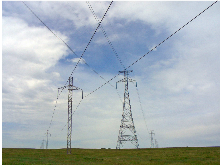
Figure C.21: HVDC long lines crossing in North Dakota, U.S.A. (United States of America, 2010. Source: Wikimedia Commons).
