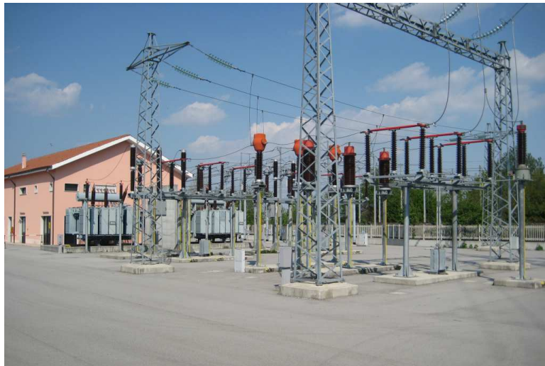
Figure 1.7: Outdoor AC side of modern 3 kV DC traction substation. (Source: Wikimedia Commons).
