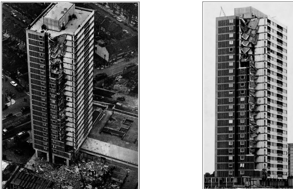
Figure 2.1 Ronan Point, evidence of the partial collapse (1968)
