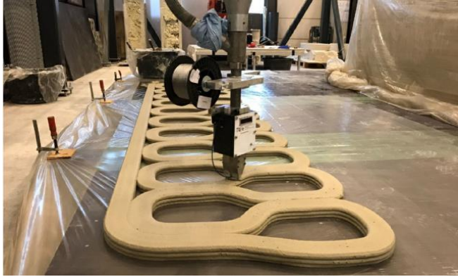
Figure 8 – Printing with the Reinforcement Entraining Device (RED) to introduce a steel cable into the concrete layer
