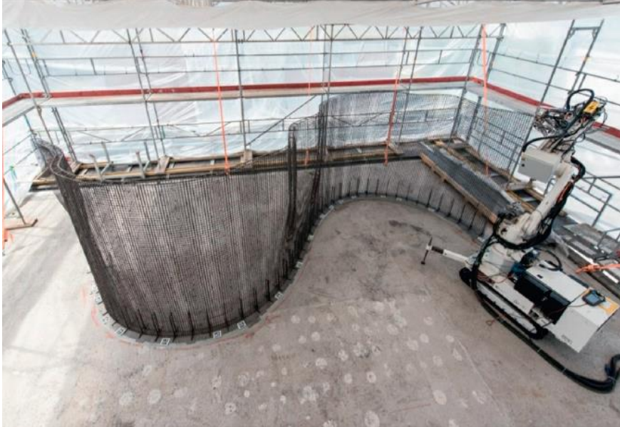
Figure 4 – Production of 14m long mesh for a double curved load bearing wall for the DFAB HOUSE, NEST building at Empa in Dübendorf, Switzerland
