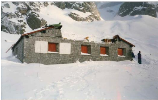
Figure 3.32 External damage (December 2000)
