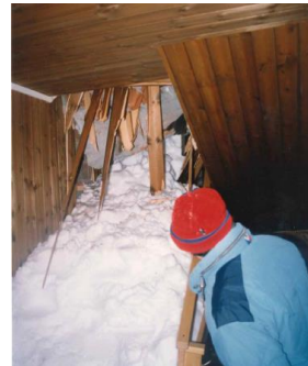
Figure 3.30 Internal damage of Bonacossa hut after the 2000 snow avalanche event
