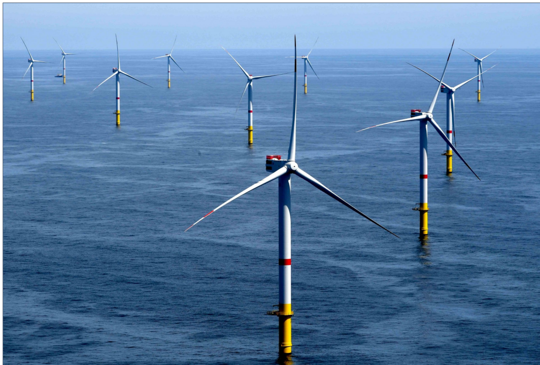
Figure 1.06 Offshore wind farm in the North Sea.
