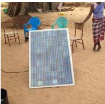
Figure 3.8. Solar panel: primary and/or back-up energy system
