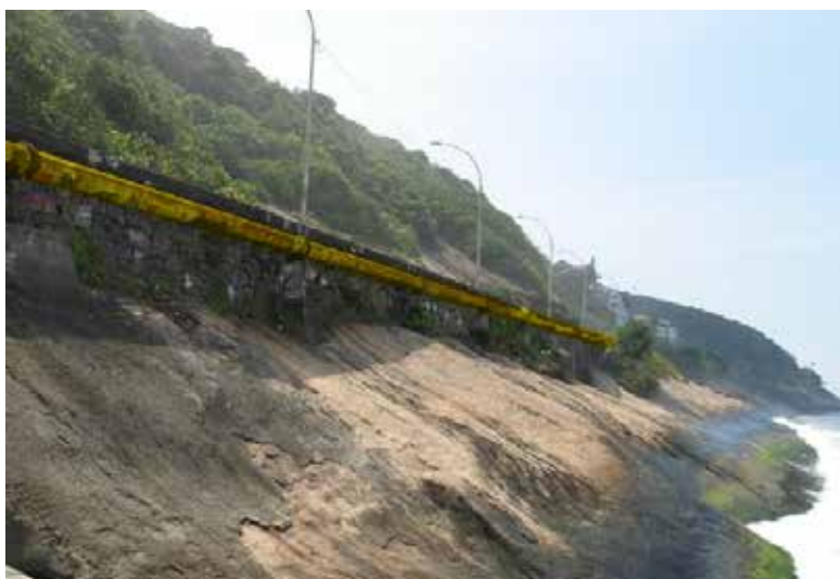
Figure 3.3.23 Main discharge pipe, Av. Niemeyer. Source: CONEN, 2012
