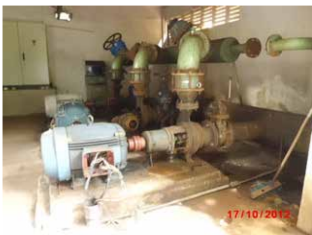
Figure 3.3.6 Water lift station EE2. Source: Planave S.A.
