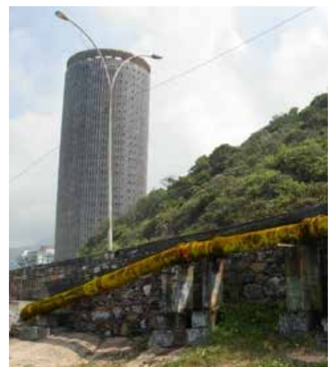
Figure 3.3.24 Main discharge pipe, São Conrado/Leblon. Source: CONEN, 2012
