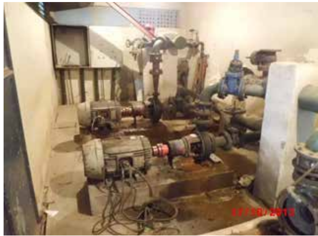
Figure 3.3.8 Lift stations EE3 and EE4. Source: Planave S.A.
