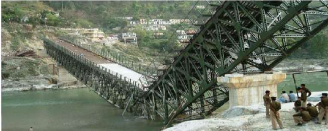
Figure 30 Chauras Bridge after failure (Failure of Chauras bridge Harshad, pabitra rajan, Pramod kumar, 2014)
