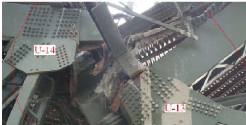
Figure 32 Intact gusset plat at joint U13 and U14 (Failure of Chauras bridge Harshad, pabitra rajan, Pramod kumar, 2014)
