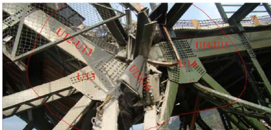
Figure 31 Joints U13 and U14 and buckled member U13U14 (Failure of Chauras bridge Harshad, pabitra rajan, Pramod kumar, 2014)
