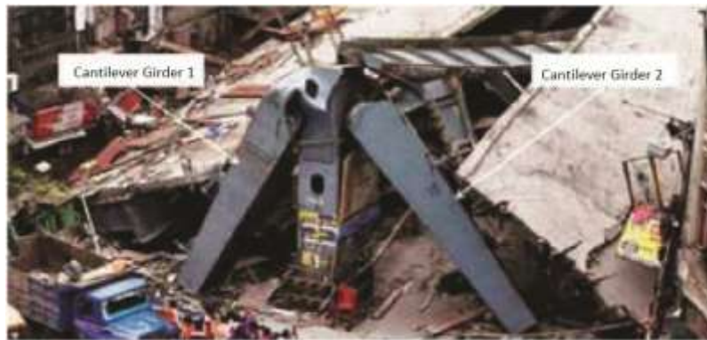
Figure 37 Collapse of the two cantilever girder (Collapse of Kolkata flyover N.Prabhakar & N.Subramanian, 2014)
