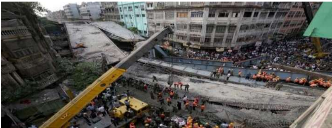
Figure 35 After failure, Concrete Deck Slab had been Laid on one Cantilever Side only (Collapse of Kolkata flyover N.Prabhakar & N.Subramanian, 2017)
