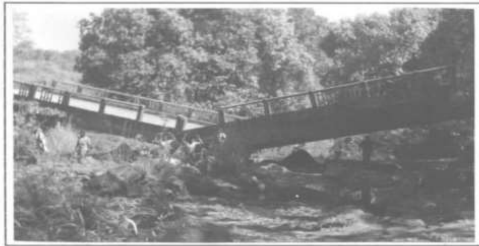
Figure 12 Langi Durg Road Bridge (Pier Failure of Bridge and Geotechnical J. K. Jain 1998)
