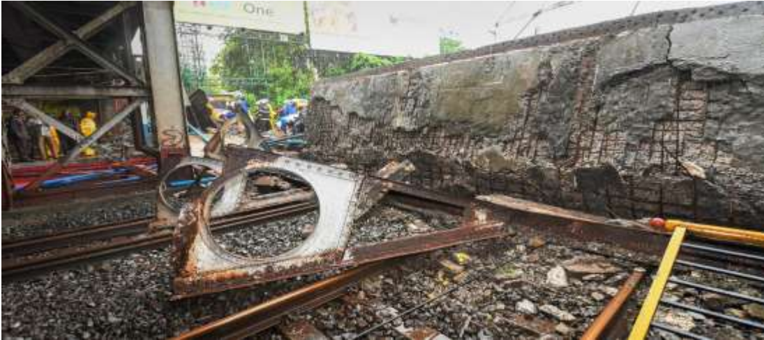
Figure 23 Failure due to corrosion – (economictimes,2018)
