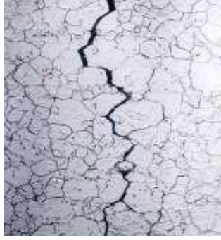
Figure 20.A Start of stress corrosion cracking. (Kamnik, April 2008)
