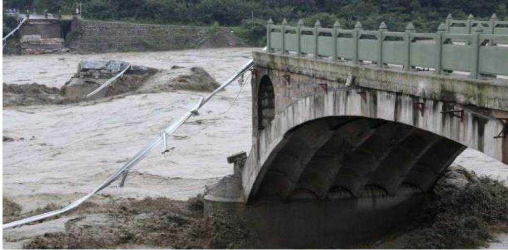
Figure 14 Collapse of Jahu Bridge – (Jahu Bridge, Pankaj, 2018)
