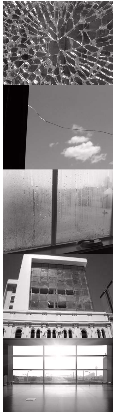
Figure 3.40; Various glazing failures of the curtain wall
