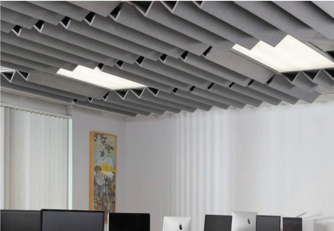
fig 65: acoustic panels on the ceiling
