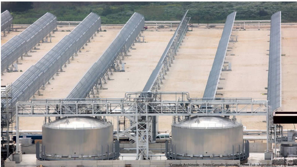
Figure 2.4: The two tanks and a part of the solar field of the ACSP plant [71]
