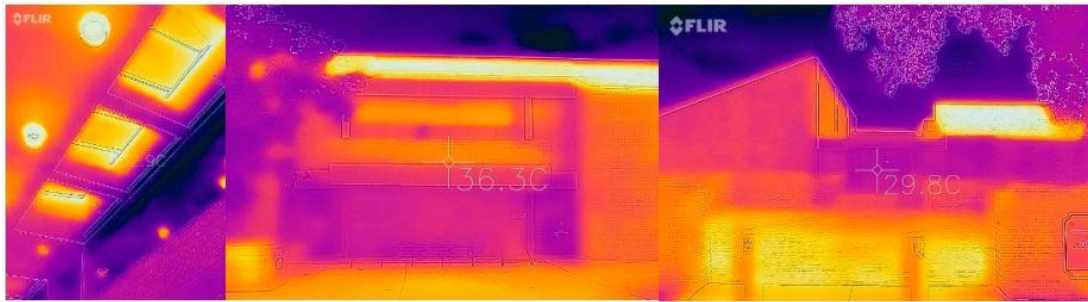
Figure 4.6. Infrared images of interior and exterior conditions [67]
