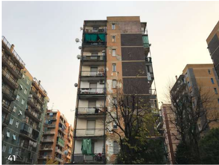
Figure 41. One of the most deteriorated facades of the critical housing block of Satellite. Source: author
