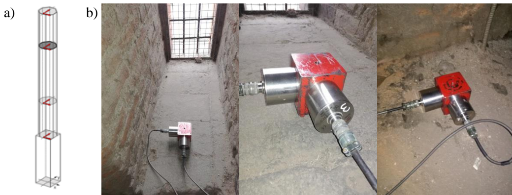
Fig. 8.6. Ambient vibration tests performed on 21/03/2017: a) layout of the sensors used for the AVT; b) biaxial accelerometers positioned in the four available levels of the tower.
