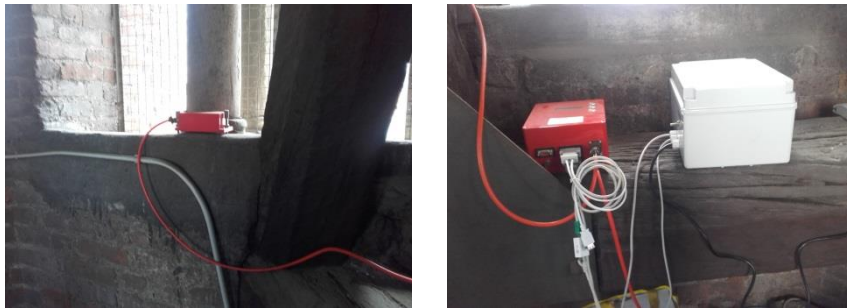
Fig. 8.3. Measurement devices installed in the San Gottardo Bell-Tower .
