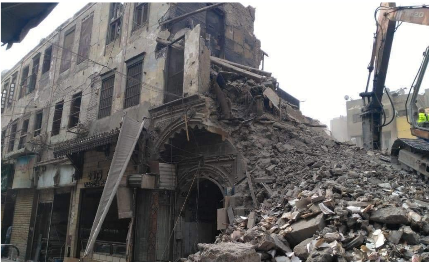
Figure (4): Wikalet Al Anbareen, located in the historic Al-Muezz Street, being demolished by the Egyptian authorities. Picture source: Al-Masry Al-Youm newspaper.
