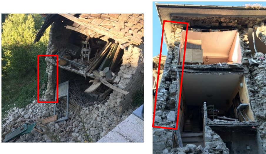
Fig. 7.1. Multi-leaf walls in two buildings located in Accumoli (RI), revealed after the collapse of the façade due to the 2016 Central Italy earthquake.
