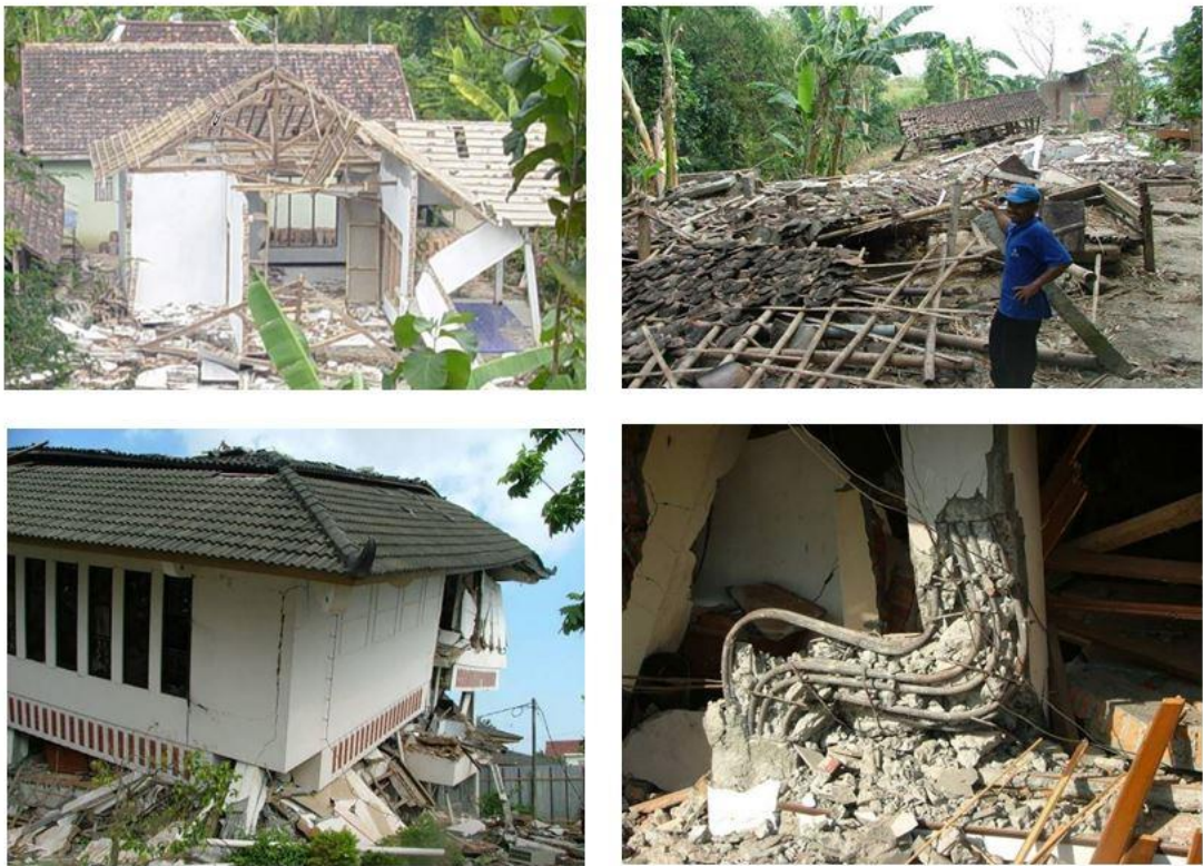
Fig. 1. 1. Severe collapses of residential building in Yogyakarta, Indonesia, after an earthquake in May 2006 [3].
