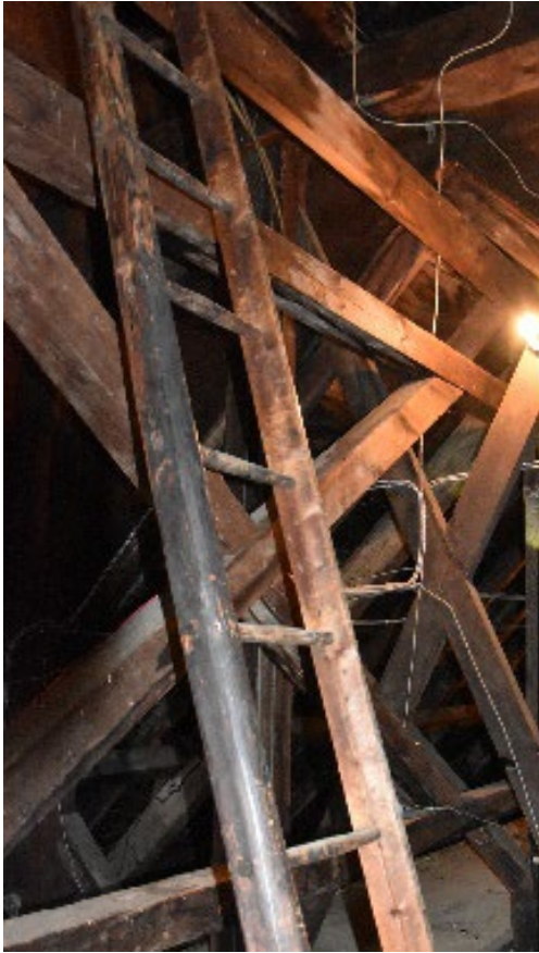
Figure 7- 40 Columns of the bell tower and brace structure of the first deck of the bell tower and longitudinal stiffening of the roof structure.
