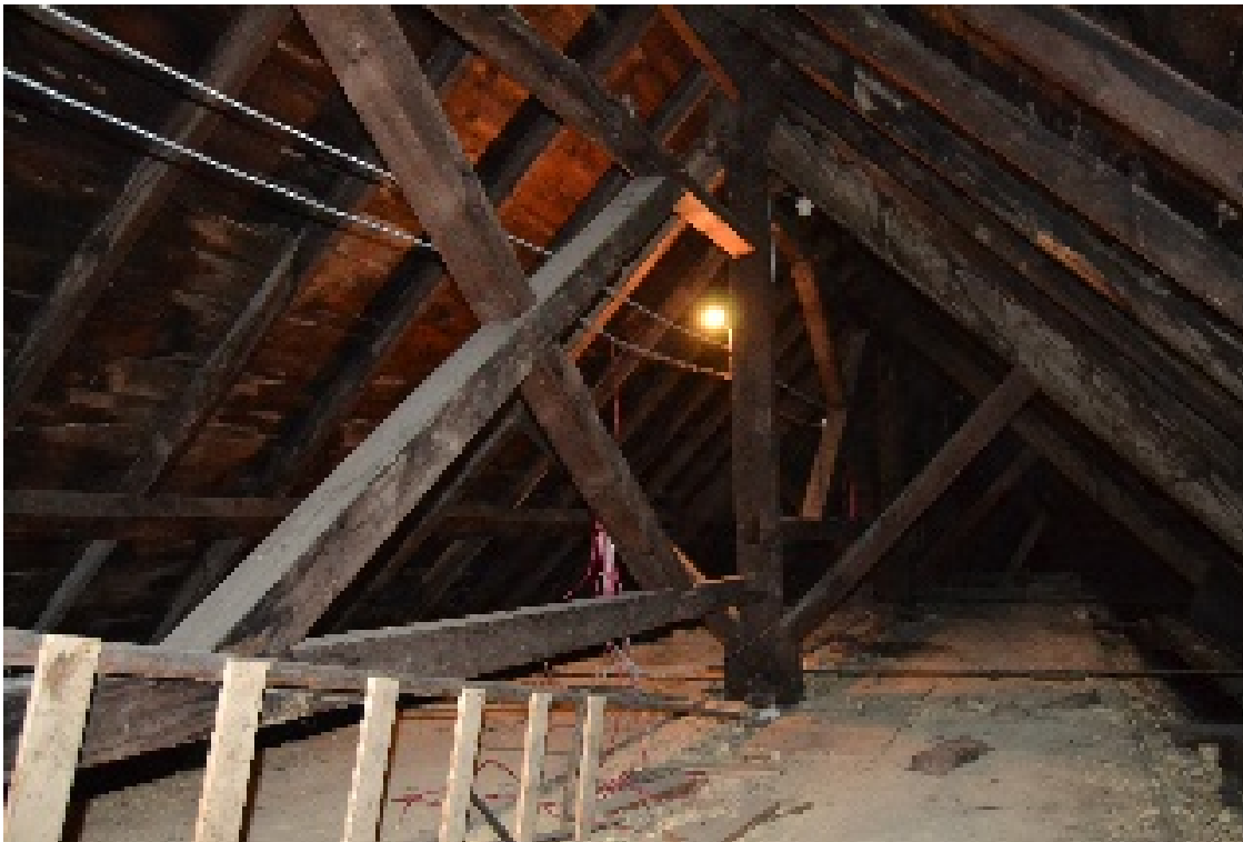
Figure 7- 42 Roof level above the central brace structure that longitudinally interconnects the trusses.
