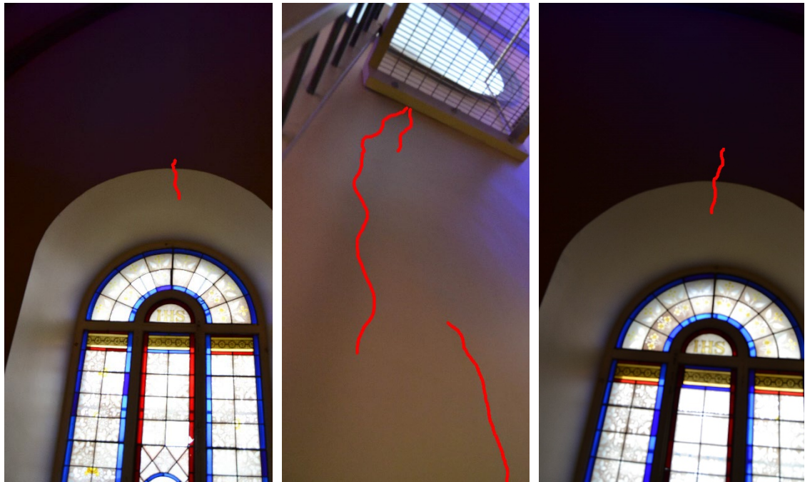
Figure 7- 21 Cracks in Sainte Famille in Boucherville: a. Rose window; b. Left opening in the façade wall at the second order; c. Below the rose window; d. Right opening in the façade wall at the second level.
