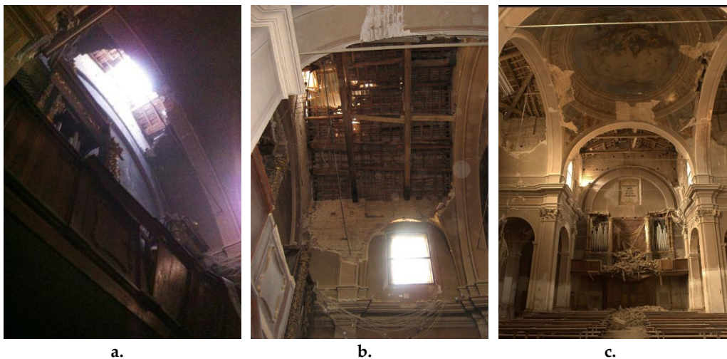
Figure 6- 5 Damage on the thin brick vaults of San Bartolomeo church in consequence of the 2012 Pianura Padana Emiliana earthquake: a. partial collapse of the vault adjacent to the façade and part of the arch after the 1st strong shock. b. total collapse of the vault adjacent to the façade, the arch, and the second vault. c. delimitation of the damage to the vaults due to the presence of the arch. Some shear damage is present in the dome.
