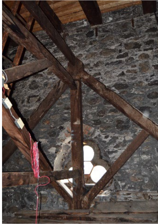
Figure 7- 41 Last truss close to the façade wall and beams of the 2nd deck of the bell tower.
