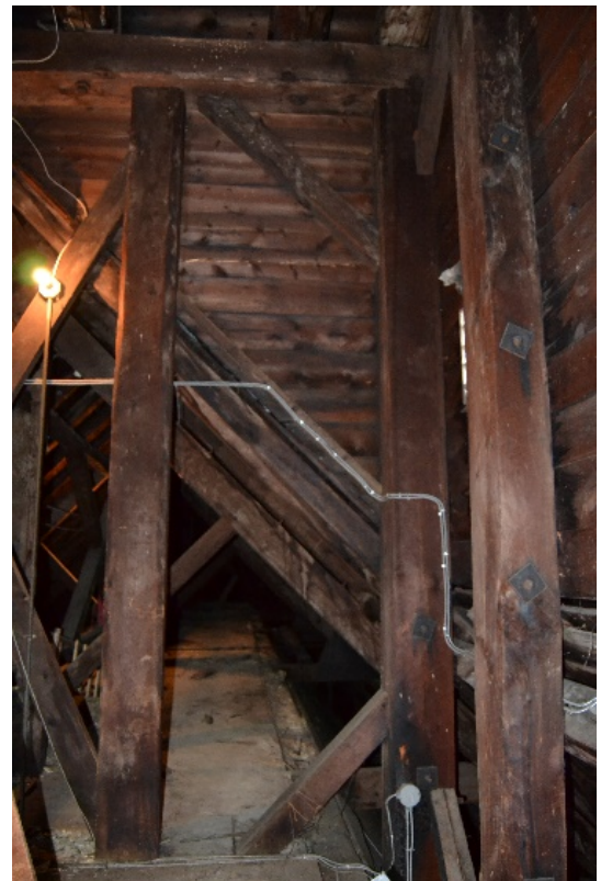
Figure 7- 39 Pillars of the first deck of the bell tower and timber structure of the first deck of the bell tower (right).
