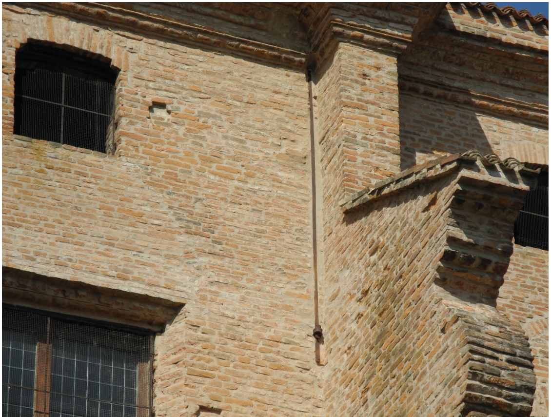
Figure 4- 8 Example of brick pattern found in one of the church sample (Superintendence of Brescia 2018).
