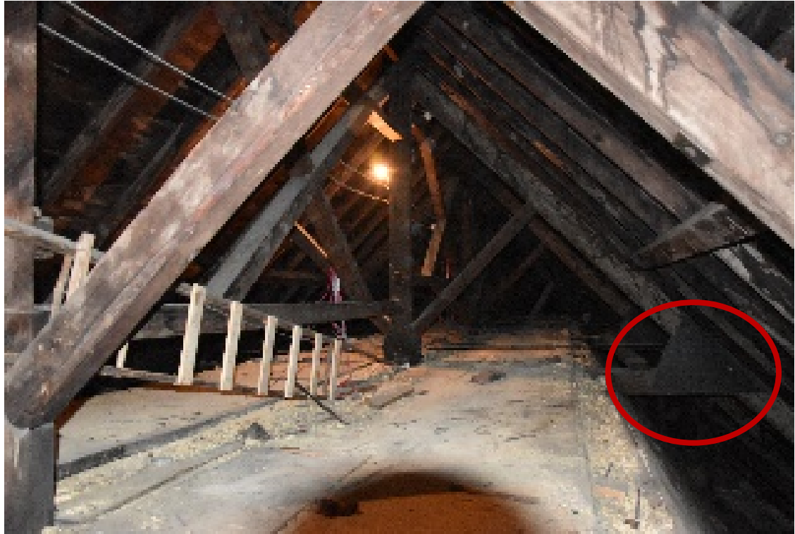
Figure 7- 43 Wider view of the roof structure: trusses and brace structure between trusses. In the background, it is visible the retrofitted truss through a metal stiffening element.
