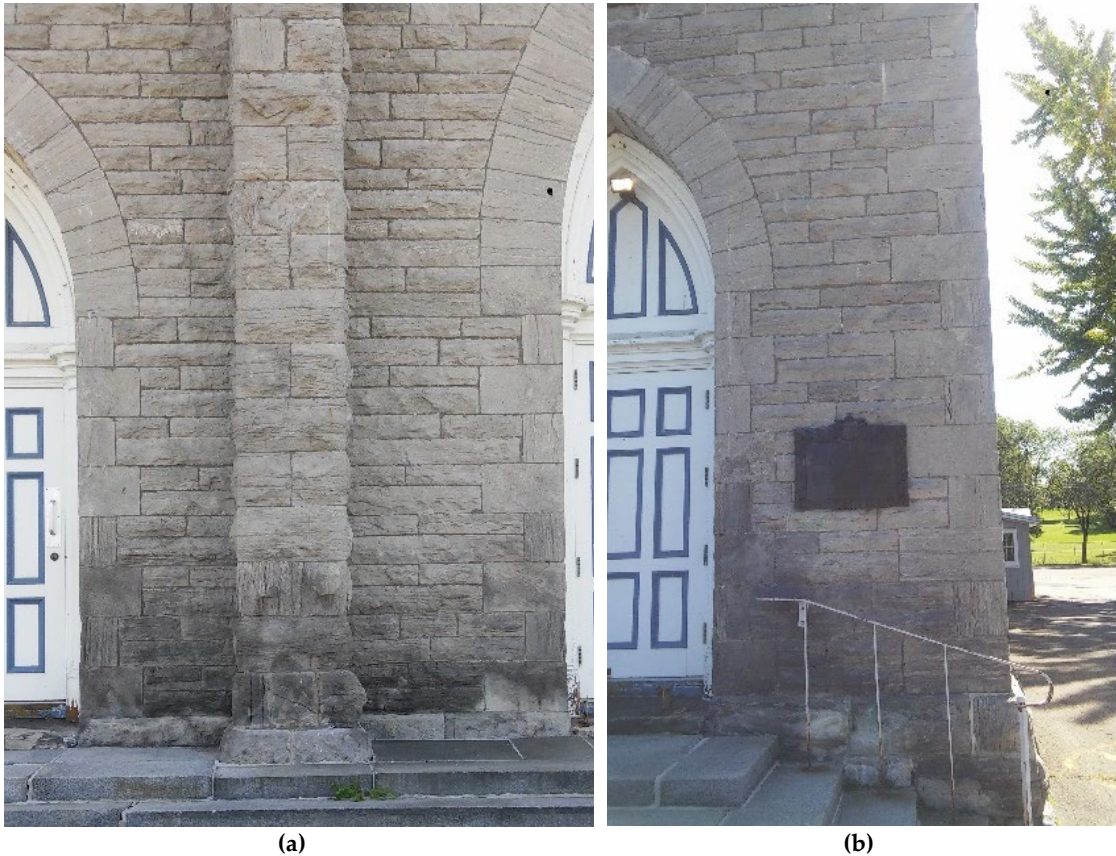
Figure 7- 48 Rising damp visible at the base of the façade: a. on the center of the façade; b. on the right corner. The photo was taken on dry season (beginning of September).
