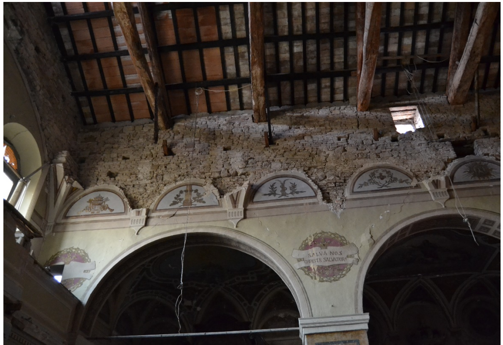
Figure 3- 9 Trusses of the roof entering the longitudinal wall of the nave. Cracks that start from the portion of the wall where the roof beams are supported.
