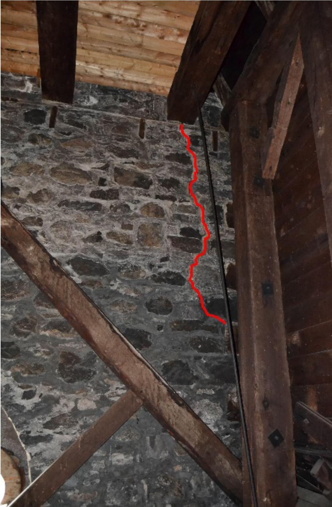
Figure 7- 52 Crack in the interior side of the façade. It has a vertical path starting at the base of one beam of the second deck of the bell tower.
