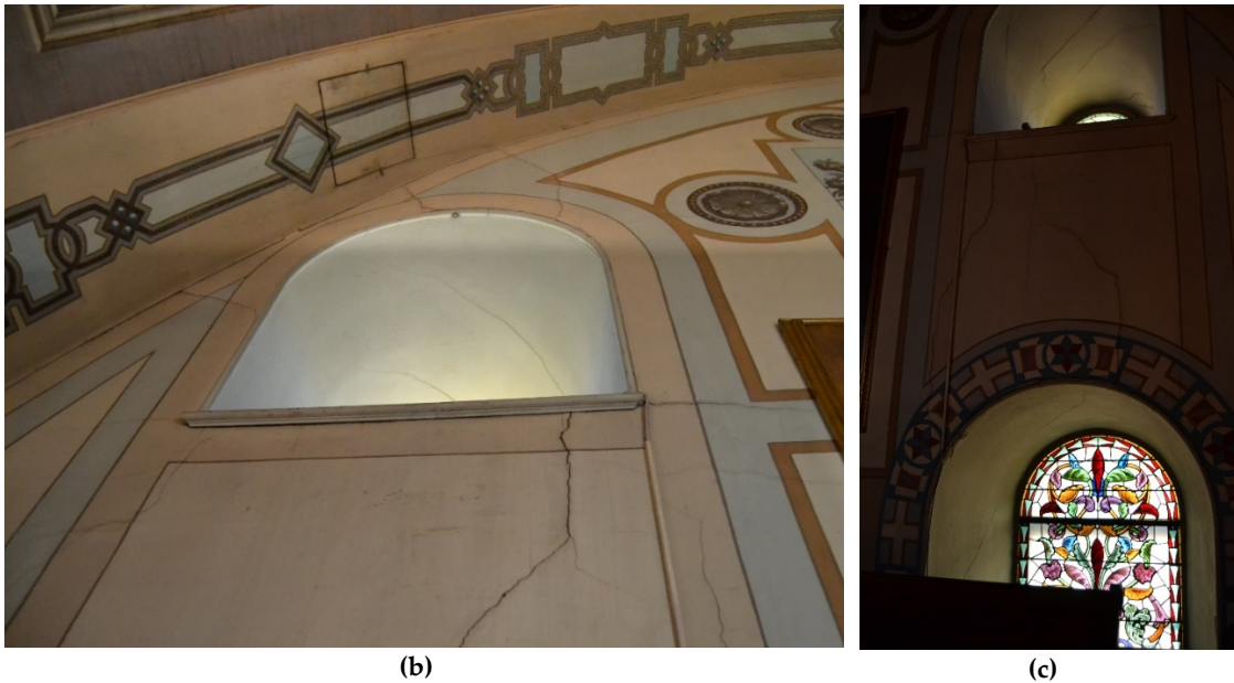
Figure 7- 22 Cracks in the façade wall of Notre Dame de Bon Secours: a. complete view towards the façade wall; b. zoom on the crack below the left opening; c. zoom on the crack above the left opening.
