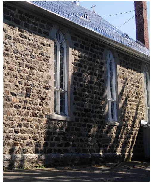
Figure 7- 34 External view of the lateral walls of the nave: roughly squared stones. The openings are marked using square blocks of stones.
