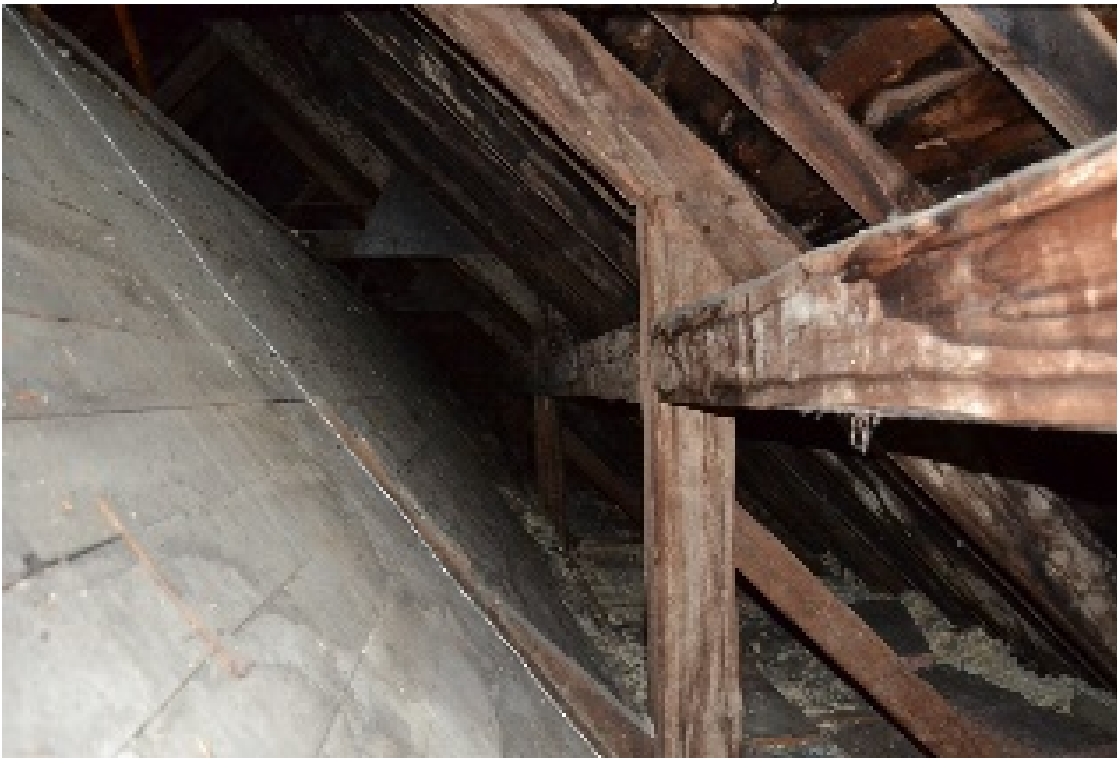
Figure 7- 46 Roof level above the lateral nave: longitudinal beams between the pillars of the colonnade. In the background the truss with the retrofitting metal element.
