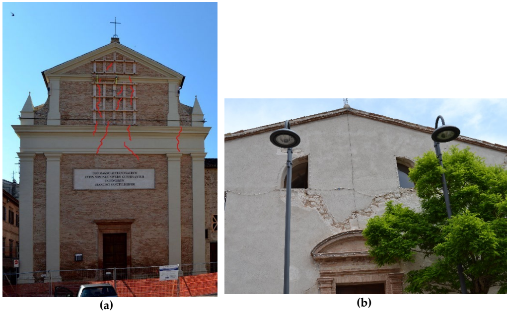
Figure 3- 7 Example of cracks in the masonry walls: a. brick wall; b. stone wall.
