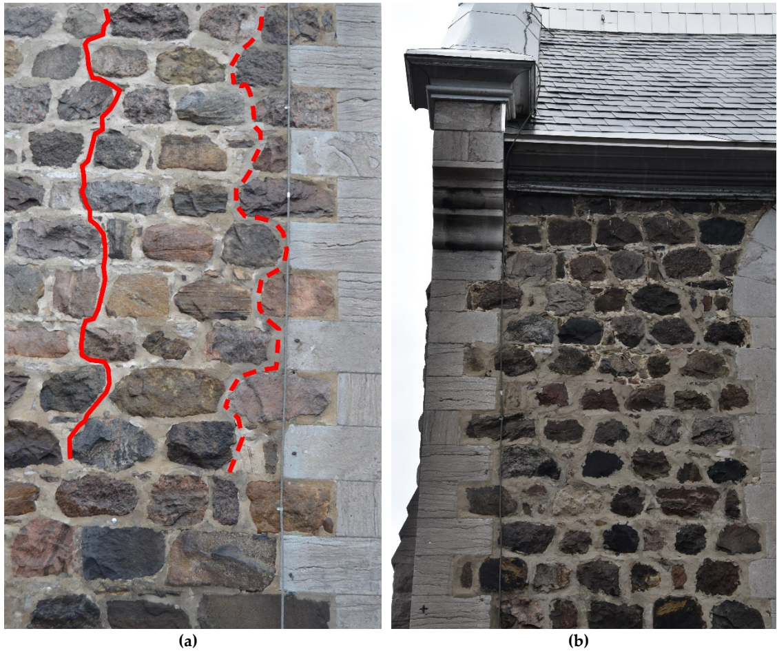
Figure 7- 50 Crack on the lateral walls of the nave: a. A vertical crack close to the corner was repaired and a new similar one appeared almost parallel to the previous one; b. A modification of the stone fabric is visible in the area close to the corner in the opposite lateral wall of the nave. A symmetrical structural problem can be assumed.
