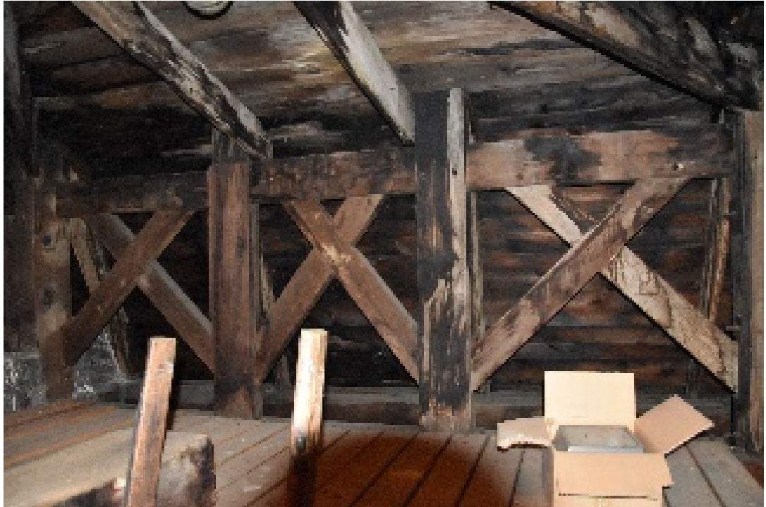
Figure 7- 37 Pillars (built in the façade wall) and brace structure between pillars at the 2nd deck of the bell tower.
