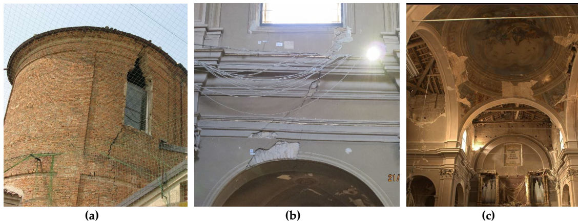
Figure 4- 21 Other damage on the church (Superintendence of Brescia 2018): a. shear cracks in the apse; b. shear cracks in the arches of the colonnade; c. collapse of other vaults of the church and damage of the central dome.
