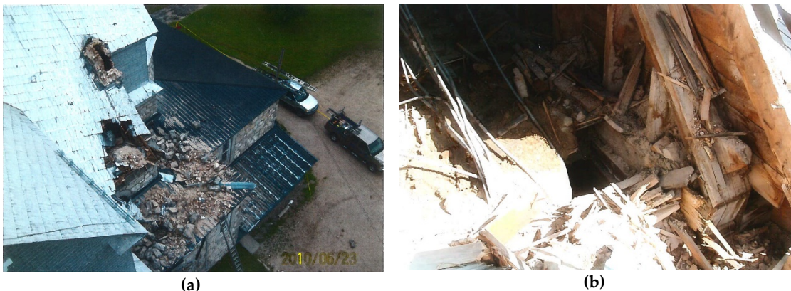
Figure 7- 7 Damage to Notre Dame de la Visitation in Gracefield: a. portion of the roof damaged by the collapse of the chimney; b. Zoom on the portion of the damage roof.
