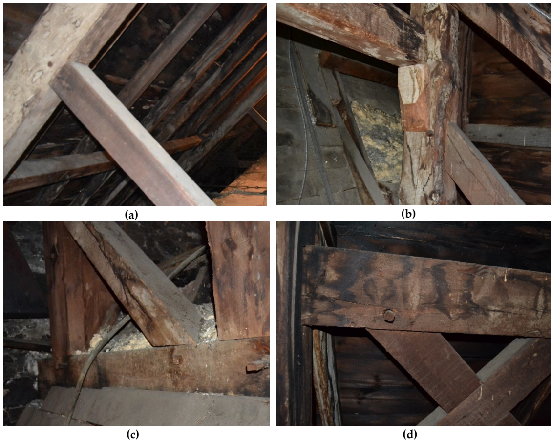
Figure 7- 53 Details of timber connections of the structure of the roof and bell tower: a. Tenon – mortise connection with timber connector between rafter and the strut of the truss; b. Tenon-mortise connection between the longitudinal stiffening structure and the column of the colonnade from the nave; c. beam of the first deck of the bell tower entering the façade and pillars of the bell tower; d. Detail and accuracy of the tenon – mortise connection between the beam of connection of the pillars of the second deck of the bell tower and the stiffening structure.
