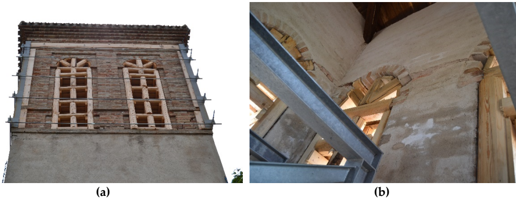
Figure 3- 11 Bell tower torsion of the upper part of the belfry of the bell tower of San Lorenzo in Dignano.
