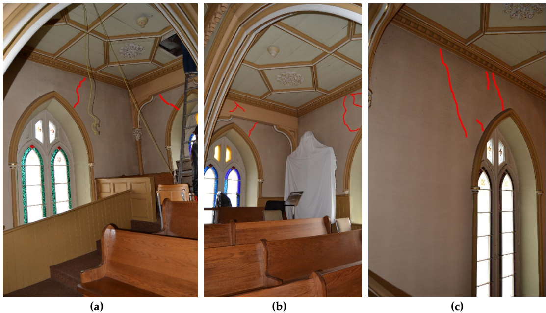
Figure 7- 51 Cracks near the openings in the lateral walls close to the façade: a. first window in the north lateral wall; b. first window in the south wall; c. second window in the south wall.
