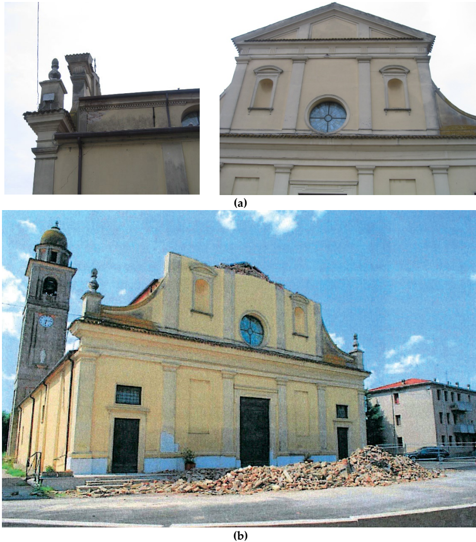
Figure 4- 5 Damage to the gable of San Giovanni Battista (Superintendence of Brescia 2018): a. Damage of the gable after the first shock (May 20), with a level of damage equal to 3 according to EMS-98 scale for Mechanism 2 (Mechanism of the gable) in the abacus of mechanisms; b. Collapse of the gable after the second shock (May 29), damage level 5.
