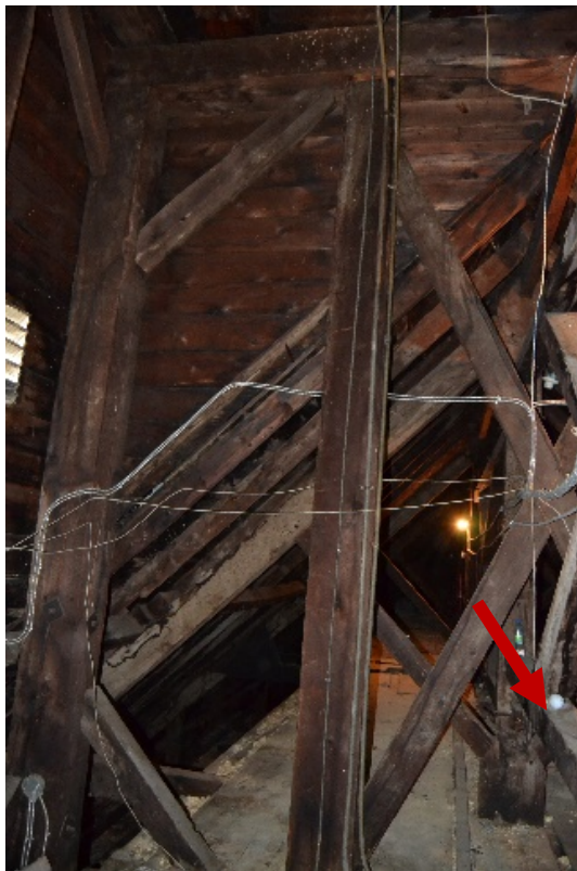
Figure 7- 38 Pillars and timber structure of the first deck of the bell tower (left).The red arrow shows the longitudinal brace structure that cross the brace structure of the bell tower.
