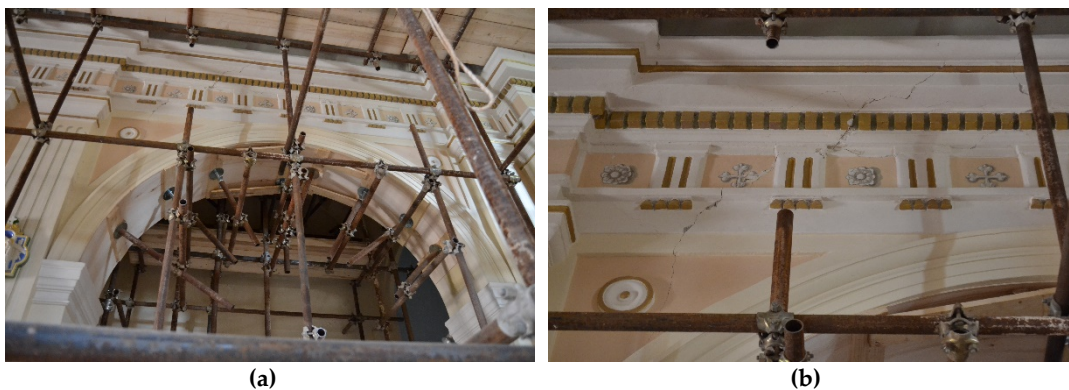
Figure 3- 8 Shear cracks in the entablature as longitudinal response of the colonnade: a. crack in the entablature of the colonnade; b. detail of the shear crack.
