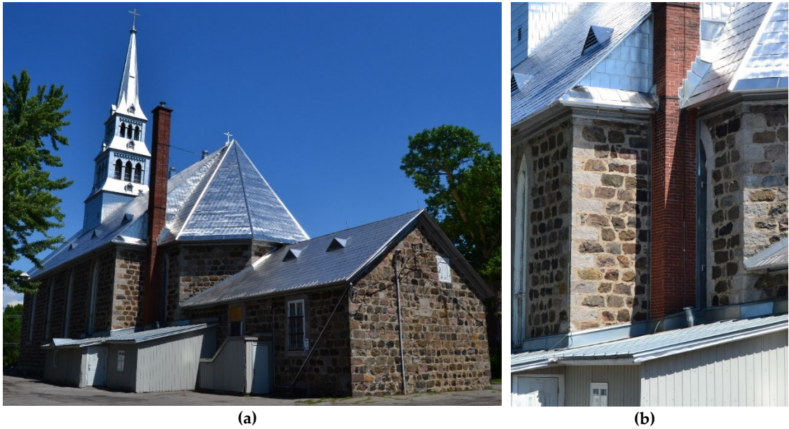
Figure 7- 47 The chimney in St. Joseph: a. Brick chimney well visible in the back of the church close to the apse; b. Brick chimney partially covers one window of the apse.
