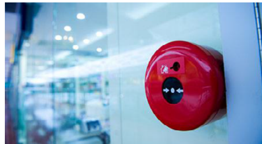
Figure 6.54 Fire alarm (Source: google)
