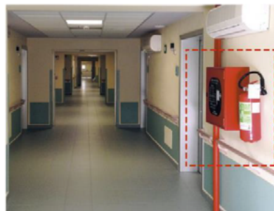
Fire extinguisher box
