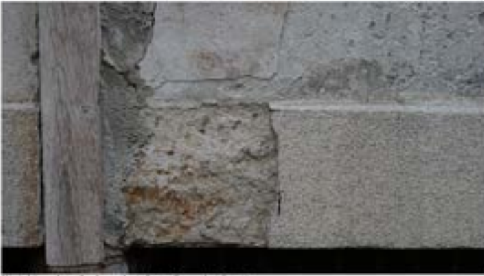
Finishing detached partly (photo from the front)
