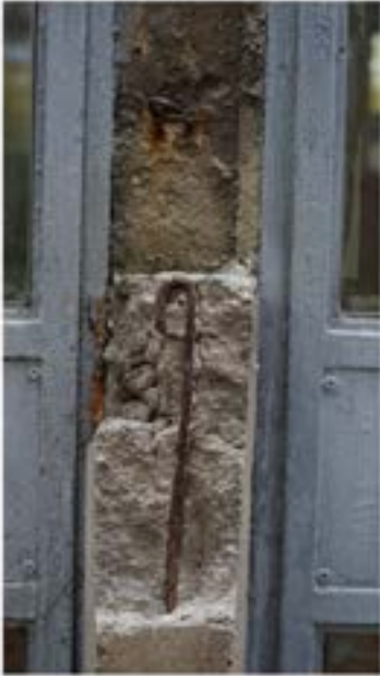
Detachment of concrete of the base(photo from the front)
