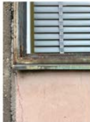
decay from the front
