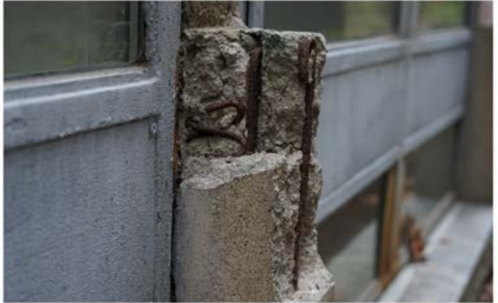
Detachment of concrete of the base(photo from the side)
