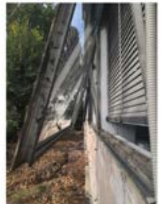
decay from the side
