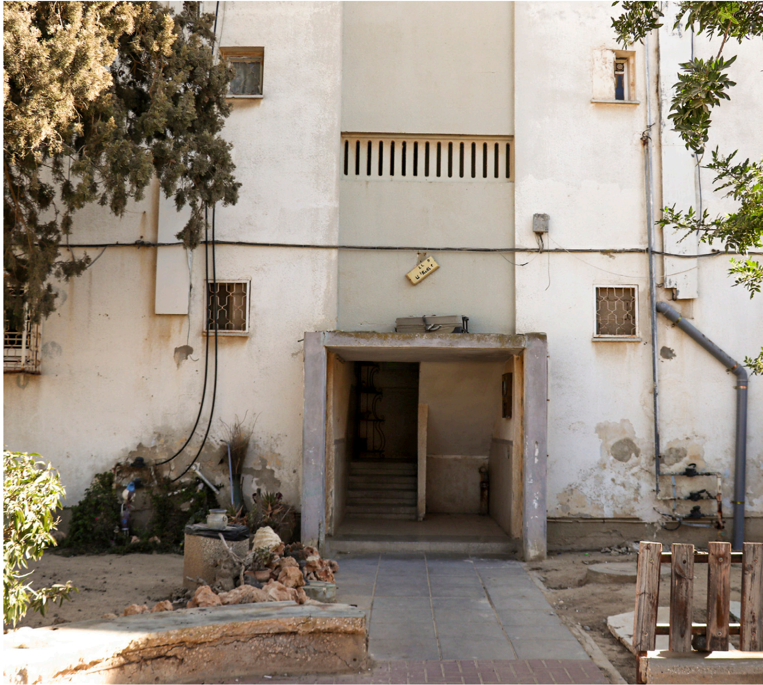
Figure178: Main facade of deteriorating structure in the Shaivat Ha Minim neighborhood. 08.2019
