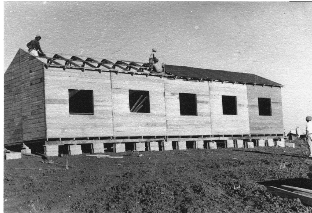
Figure 67-68: Constructing the Swedish sheds in Dimona. Unknown photographer, Unknown year. In: The Tuvyahu archive of the Ben Gurion university library, Photo No. 02156, 02157
