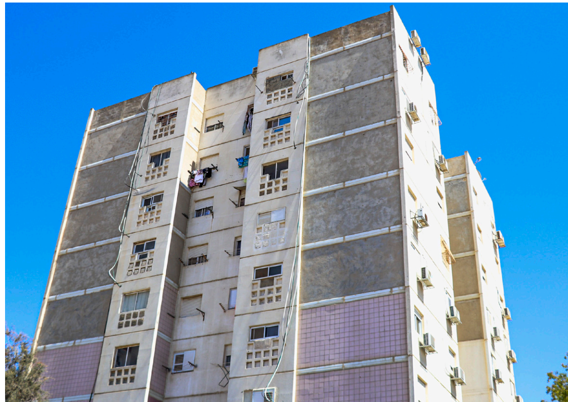
Figure 164-165 :Wetness at the exterior wall and absence of ceramic tiles at the external facade in Khahmei Israel neighborhood. 08.2019
