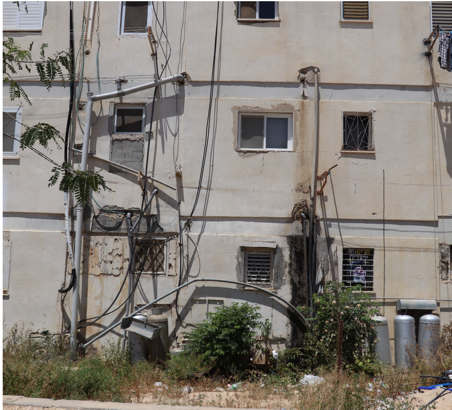
Figure 161: Deteriorating structure in Yoseftal neighborhood. 04.2020
