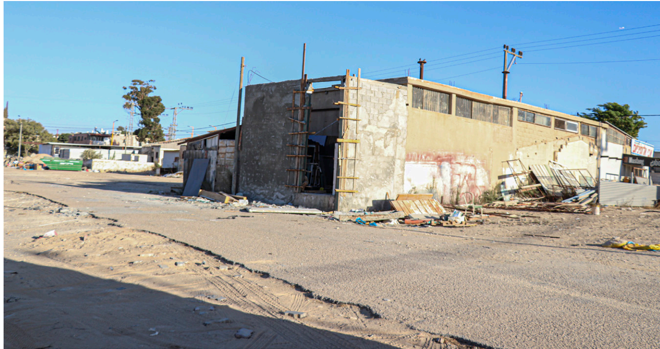
Figure 158: abandoned structure that had been penetrated by invaders in the heart of the Shivat Haminim neighborhood. 08.2019
