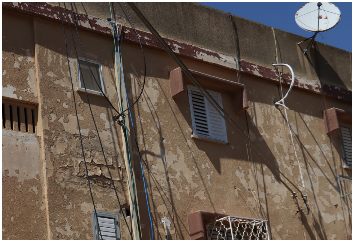
Figure 162-163: Deteriorating structures in Yoseftal neighborhood. 04.2020
