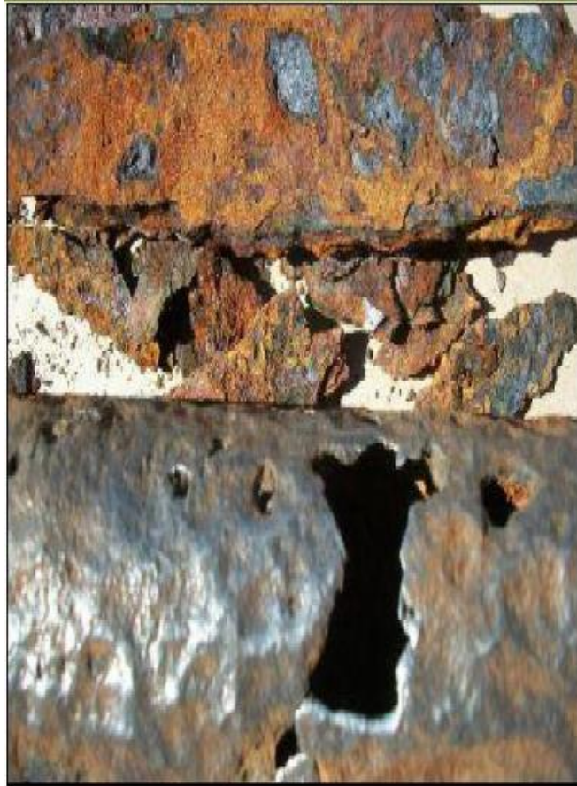
Figure 14: damaged pipeline caused by internal corrosion [16]
