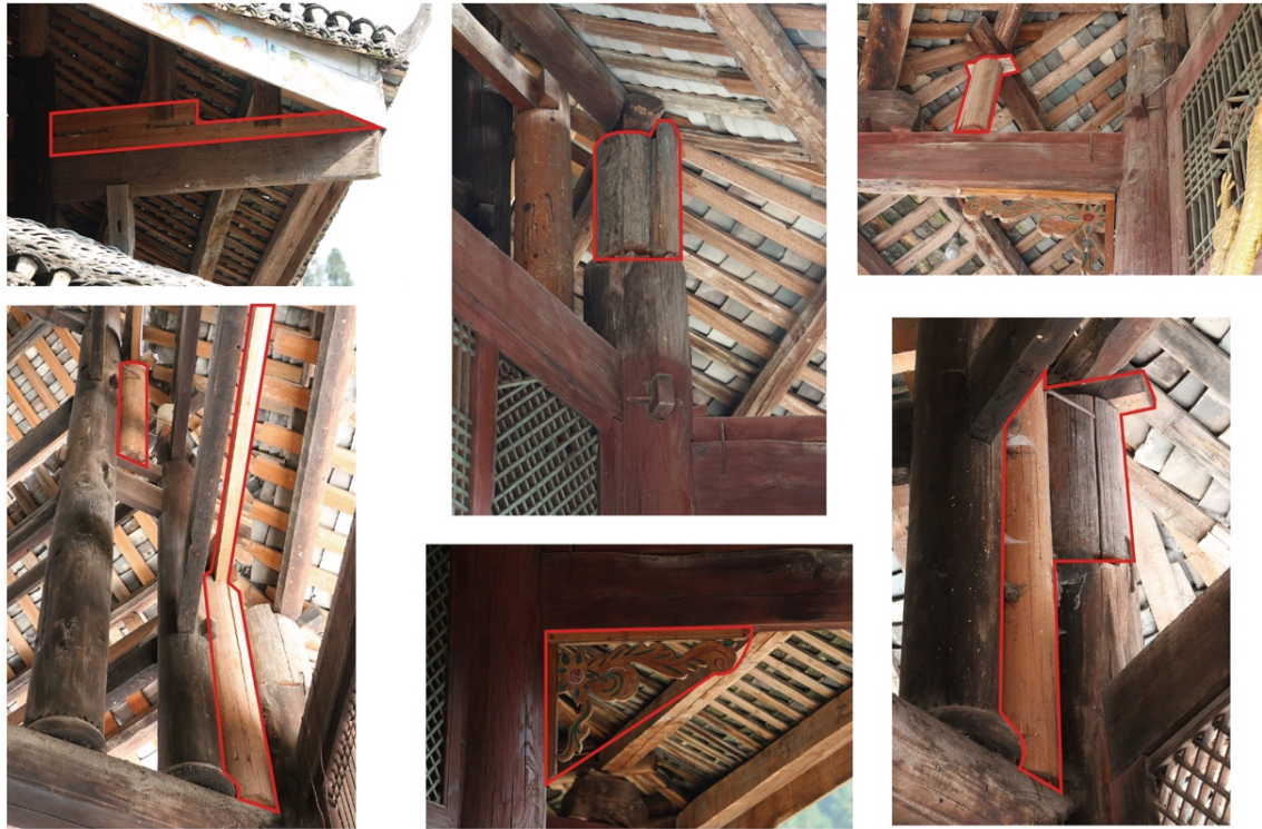
Fig. 3-17 Inappropriate additions of Zengying Drum Tower marked in red lines
