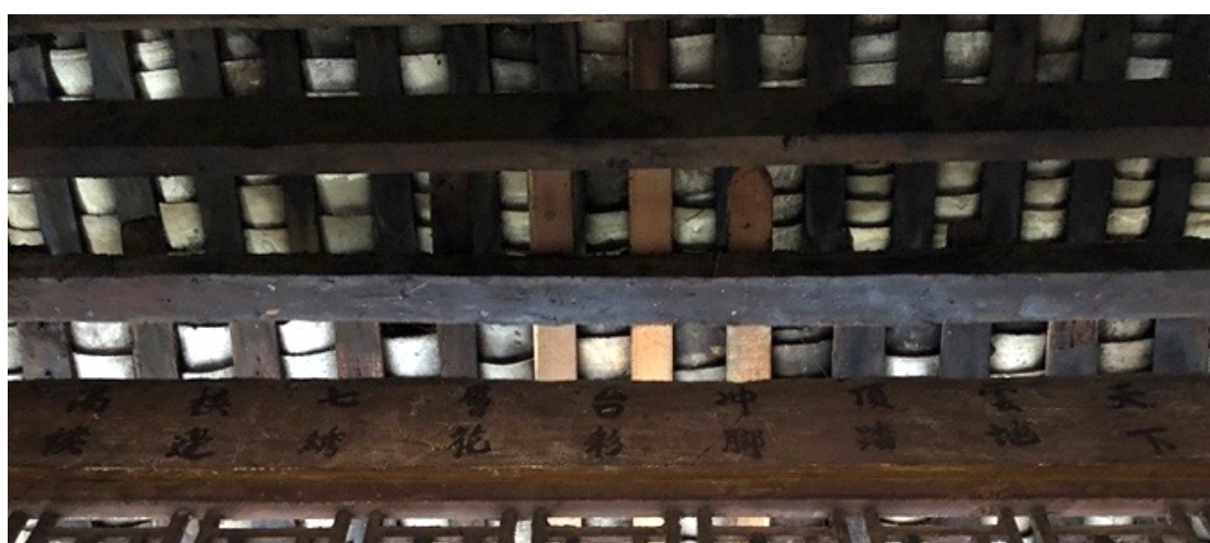
Fig.3-21 The old and new elements are visually distinguished in Zengchong Drum Tower
