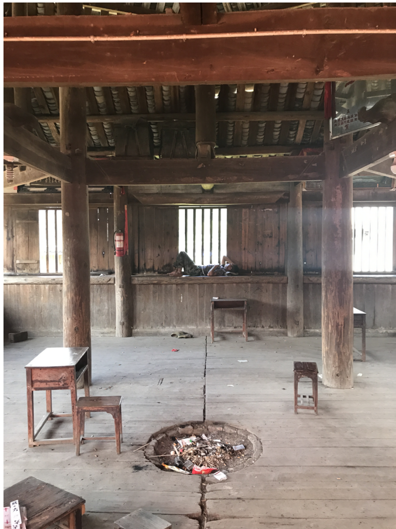
Fig.4-11 Combustible materials around fire-place (Photograph by Francesco Augelli, 2017)
