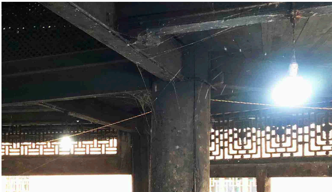
Fig.3-6 Aged and disorganized electrical wires (Photograph by author, 2018)
