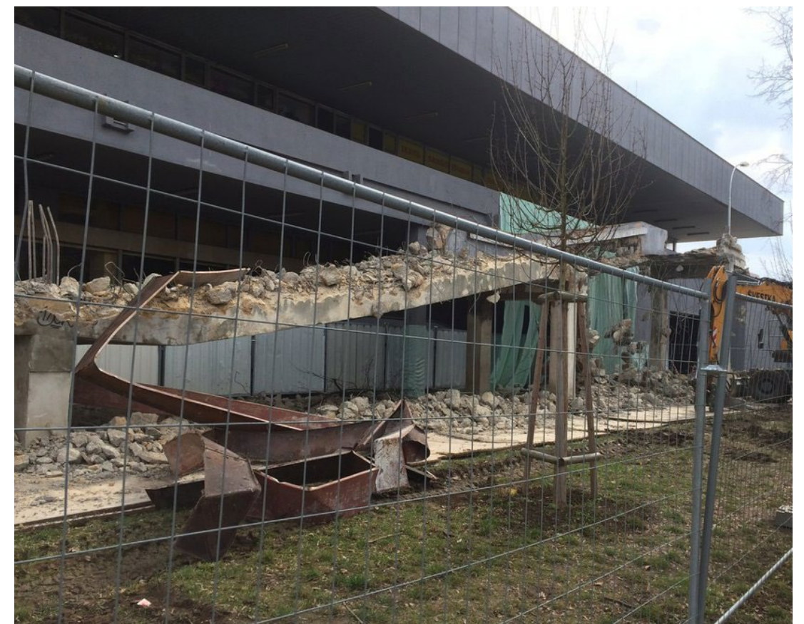
Fig. 43. Demolition of staircase arose a wave of nostalgia among inhabitants. © Daniel Vitouš, 2016. Source : https://www.blesk.cz/galerie/regiony-praha-praha-zpravy/628822/oc-odra-v-bohnicich-prislo-o-betonove-schody-podle-majitele-je-nikdo-nevyuzival?foto=7
