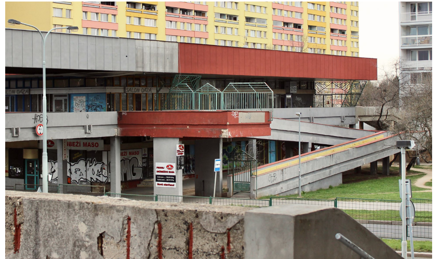
Fig. 28 East facade with closed ramp and closed portico in the first floor connecting the terrace of apartment building. © Rudolf Nikerle
