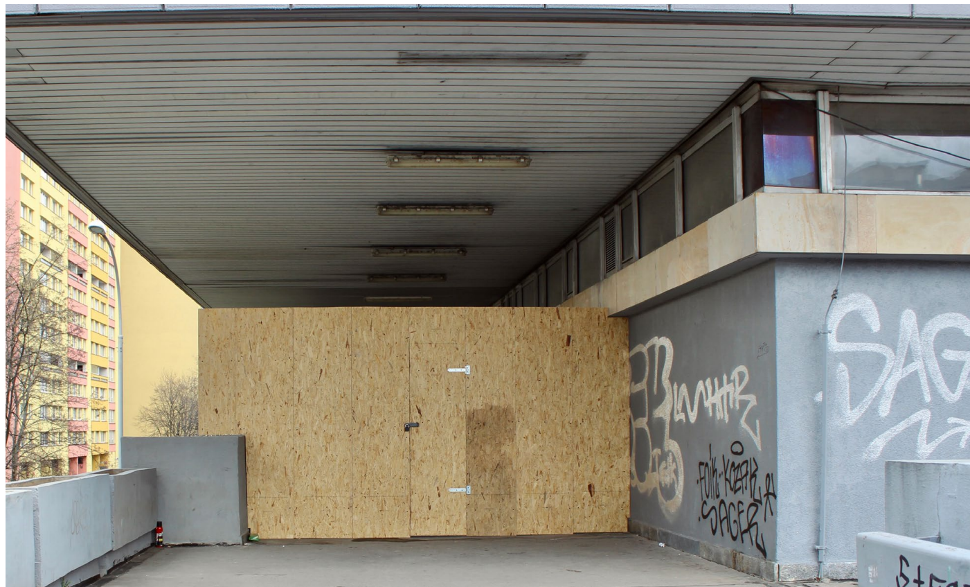
Fig. 27 Blocked portico in the first floor. © Rudolf Nikerle
