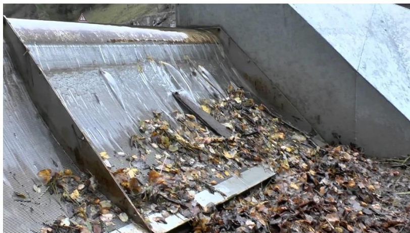
Figure 4.1: Example of a clogged intake
