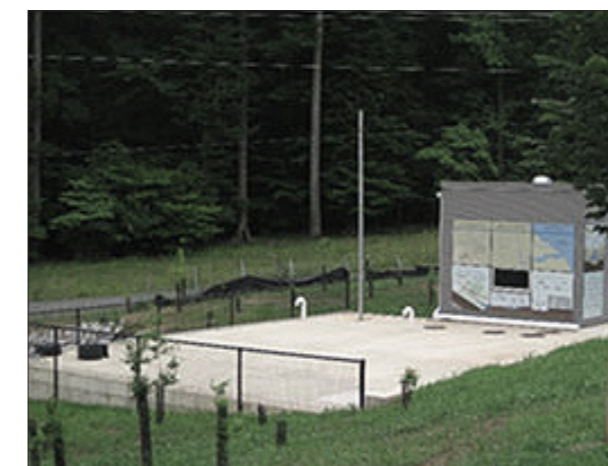
Figure 77. Pump House, used as an outdoor classroom © Rainwater Management Solutions
