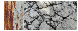
Figure 15&16. Close-up of rusty metal surface with corrosion patterns and texture; High angle view of cracked and weathered concrete pavement texture.
