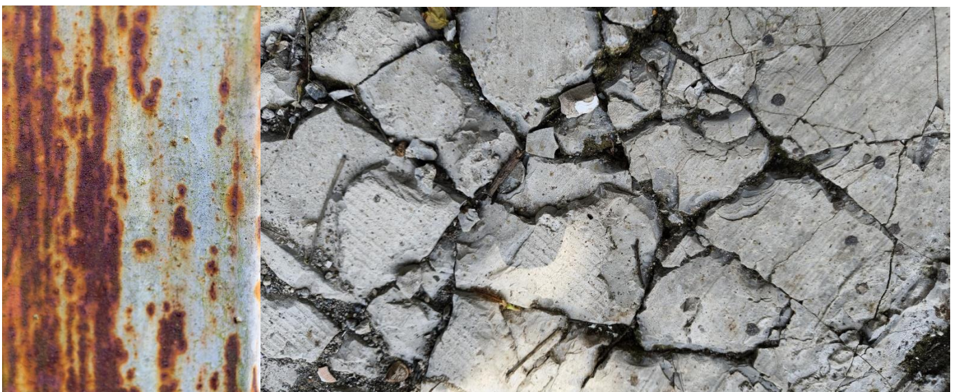
Figure 15&16. Close-up of rusty metal surface with corrosion patterns and texture; High angle view of cracked and weathered concrete pavement texture.
