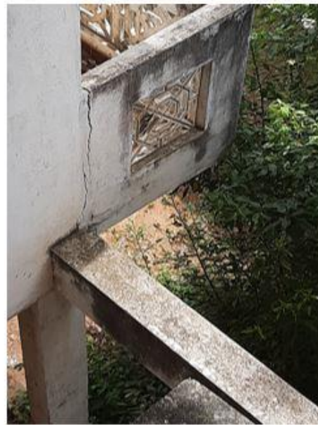
Balcony Parapet Crack
