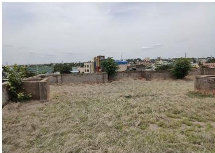
Figure.17. Grass and tree growth on the terrace
