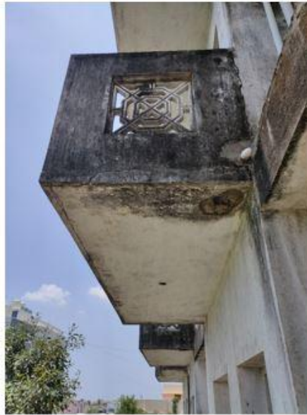
Balcony Slab Crack
