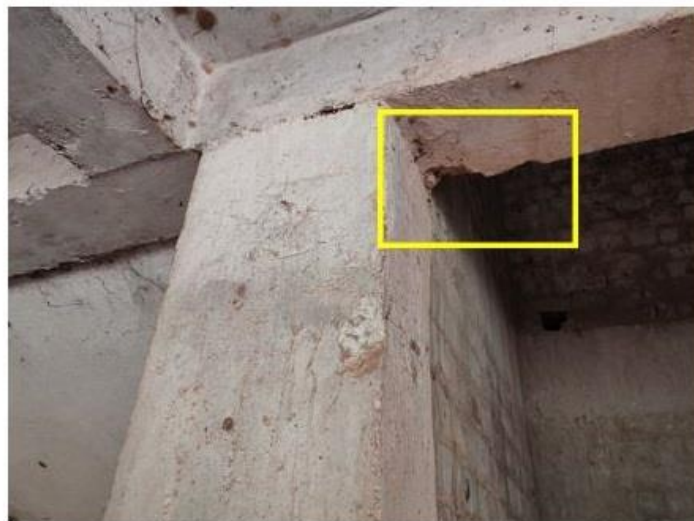
COLUMN AND BEAM JUNCTION CRACK
