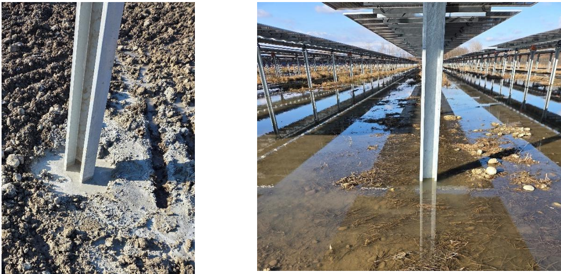
Figure 23 - Foundation part of plant of Vercelli
