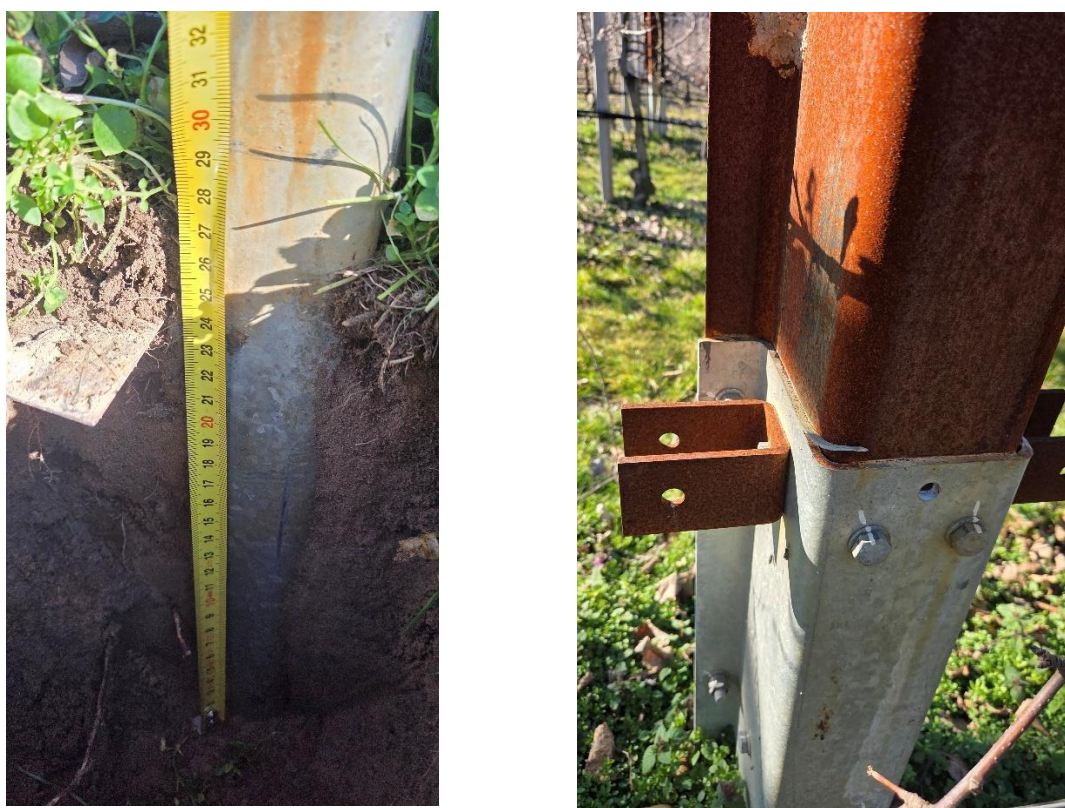
Figure 28 - Buried part and connection joint of plant of Ora
