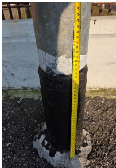
Figure 37 – Bituminous protection of illumination pole
