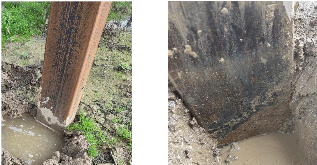
Figure 22 - Buried part of plant of Modena
