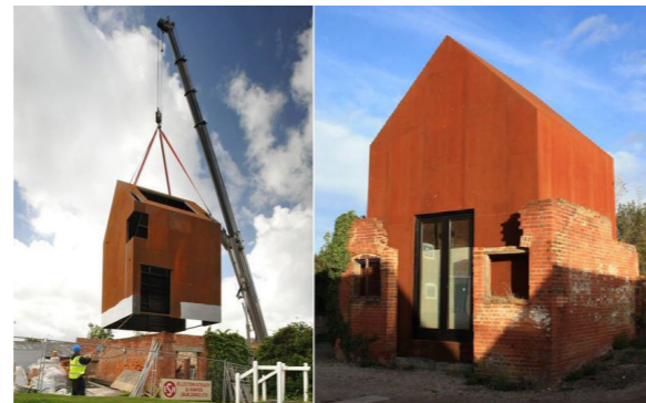
Figure 44: Dovecote studio By carefully placing a prefabricated steel home into the stabilized crumbling ruins of the old dovecote, the one-story brick building was converted to serve as an artist's studio.
