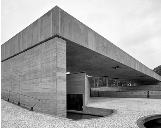
Fig. xx: Picture of the reinforced concrete slab of the Brazilian museum of Sculpture
