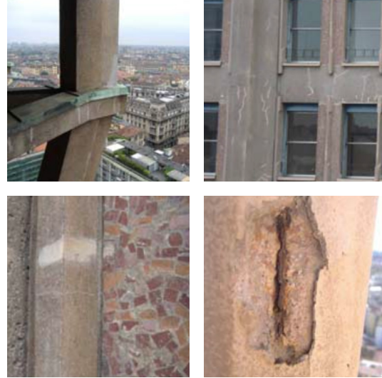
Fig. xx: Pictures showing some detected decays on the structure and elements made of reinforced concrete
