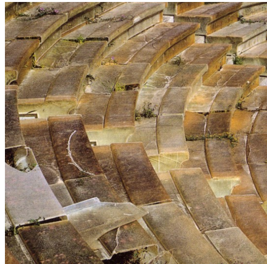
Fig. xx: Picture showing the condition of the cover: yellowing and spontaneous growth of vegetation
