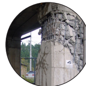
④ Collapse of the structure
