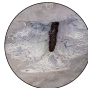
③ Concrete cover detachment
