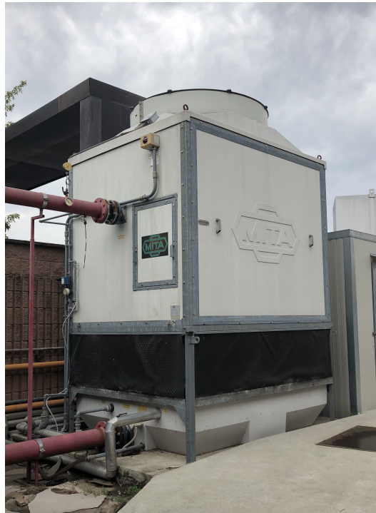
Figure 2.18: Wet cooling tower
