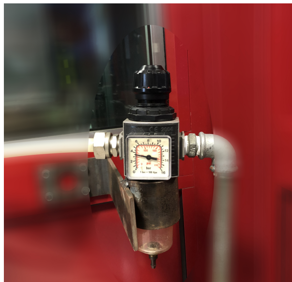
Figure 5.12: Compressed air valve at test bench
