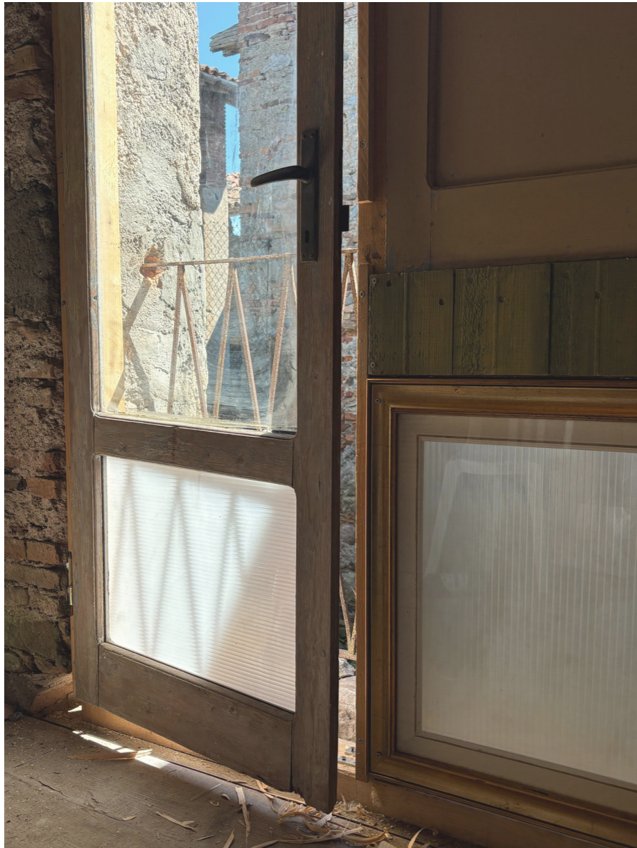
The subtle play of light between the semi-transparent panel and the shadow of the original railing
