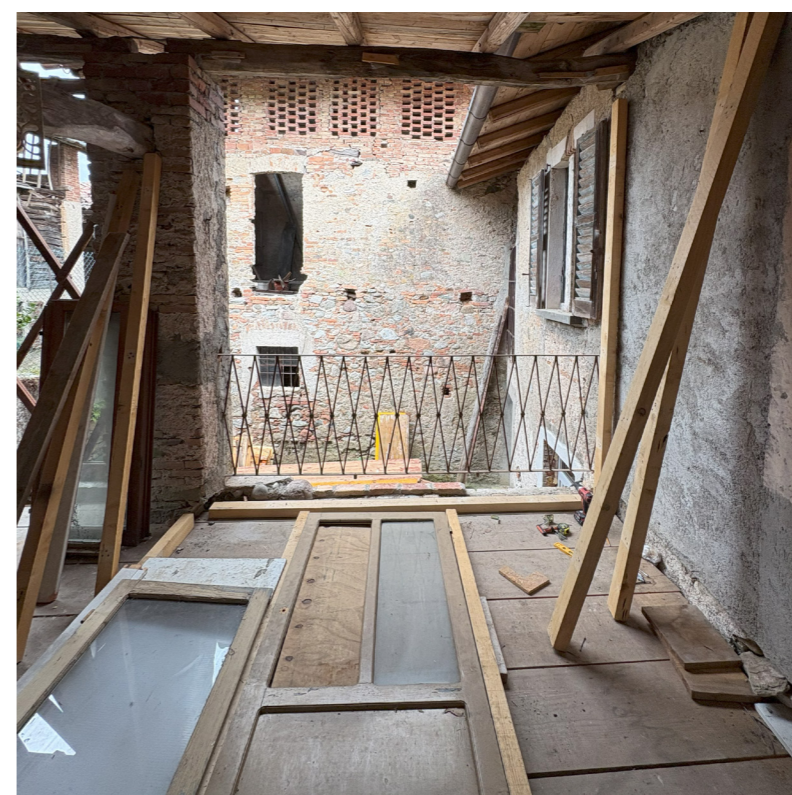
Checking the configurations directly on the floor, allowing small nuances to help us improve the arrangement
