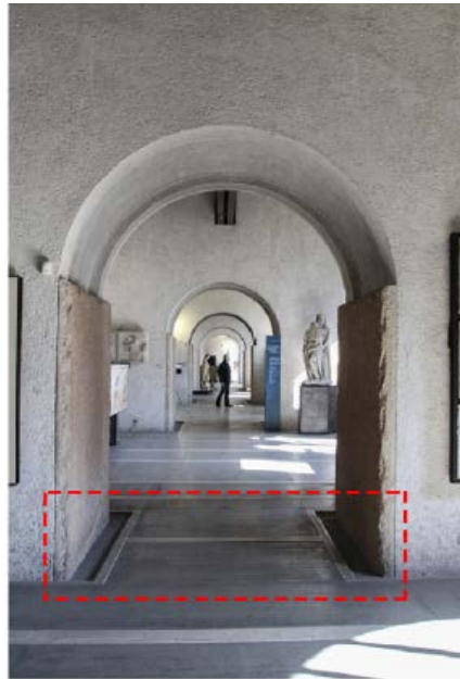
Fig. 04.39: Gap between the existing and new flooring, gallery
