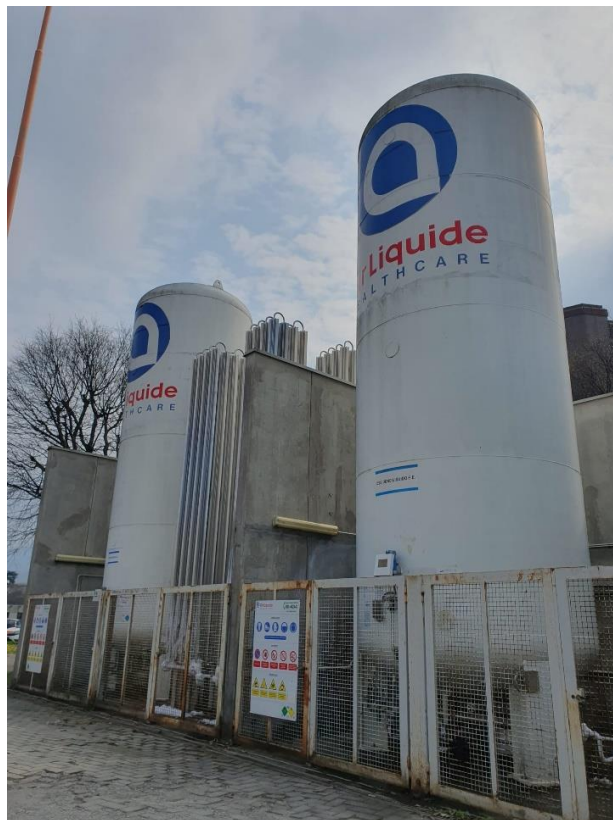
Figura 1.13: Serbatoi gas medicale
