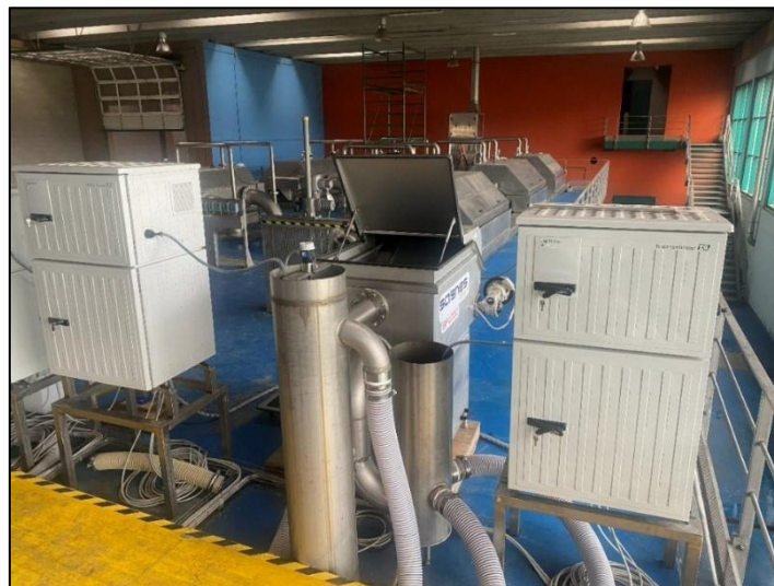
Figure 15: View of the Belt demonstration-scale filtration pilot plant installed at the Lariana Depur WWTP.
