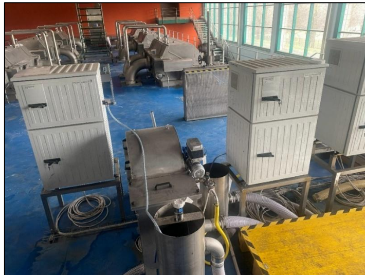
Figure 12: View of the DISC demonstration-scale filtration pilot plant installed at the Lariana Depur WWTP.
