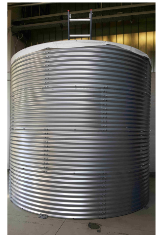
(b) The prototype tank inside B6 labs after test installation.
