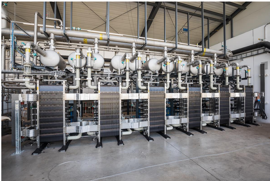
Figure 1.7 – Picture of the H2FUTURE PEM electrolysis system
