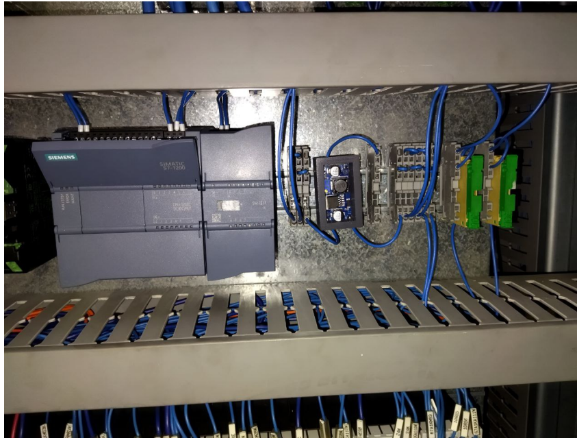
Figure 6.3: The PLC system installed in the electrical panel
