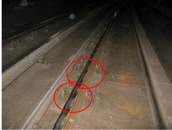
Figure 1.2: Track affected by corrugation.
